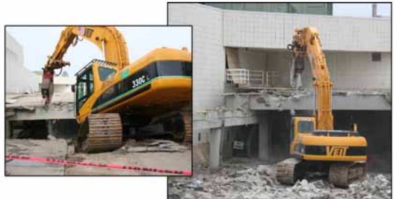
Removal of the upper parking deck on the Wallace Building's north side raised dust and a lot of questions.
