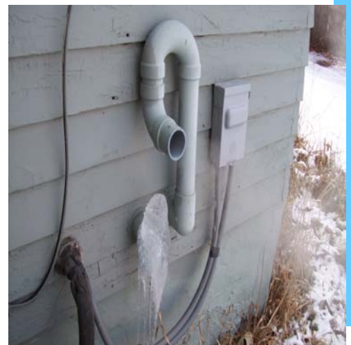
This furnace exhaust is plugging the intake when the condensation freezes.
