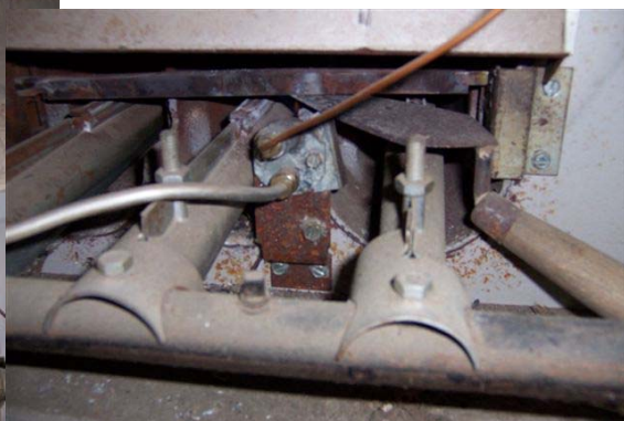
Notice the cement trawl used as a deflector...
