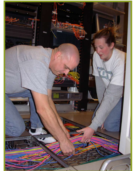
AJ Wineski and Shanna Wylie bind color-coded network cables in the IDPH Data Center in the Lucas Building.
