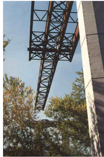
The cantilever support condition during the third launch from Pier 4 to Pier 3
