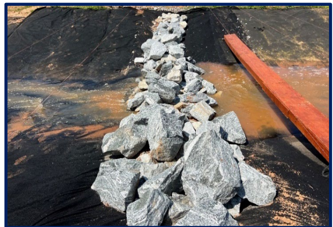
Iowa DOT Standard rock check dam
