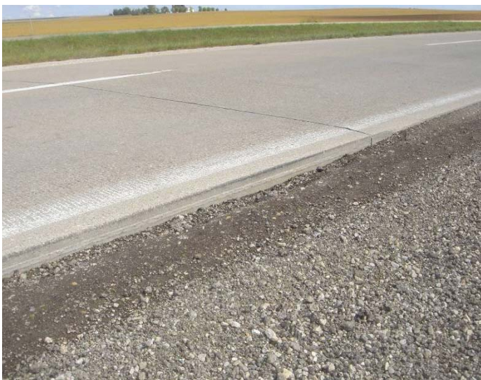
Edge drop-off along the outside shoulder caused by vehicle off-tracking
