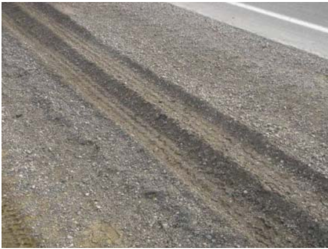
Performance of the fly ash–stabilized shoulder section after seven months: stabilized section (top) and control section (bottom)
