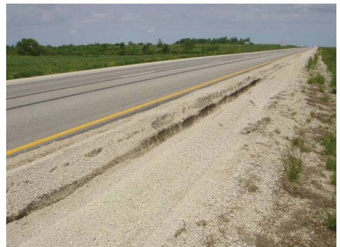
Severe shoulder rutting caused by bearing capacity failure of the soft underlying subgrade
