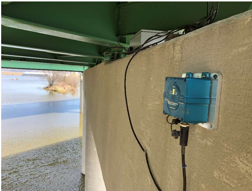
Figure 4. Photograph of SENSr System Deployed on I-29 Bridge
