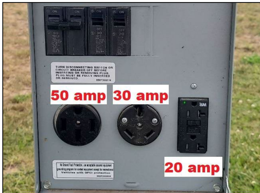
Photo of the electricity box
