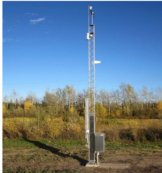
Figure 1.1. Typical stationary RWIS station
