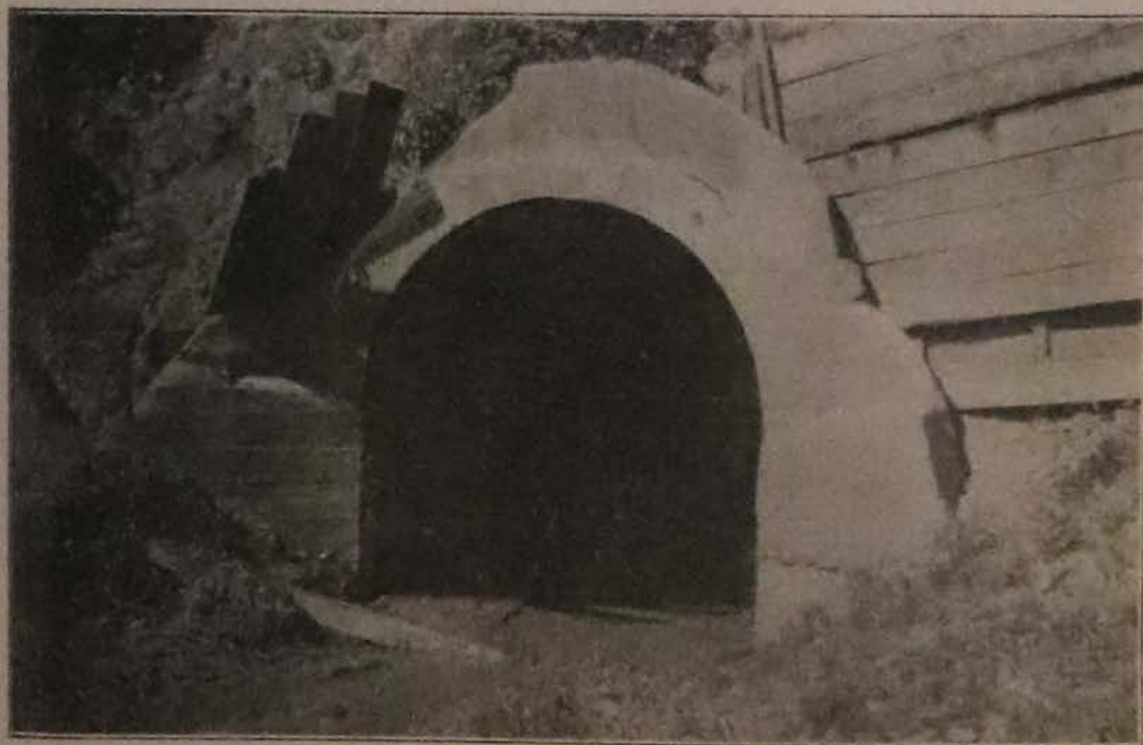
Fig. 36—Failure of Spandrel and Wing Walls on 12 foot Sub Culvert
