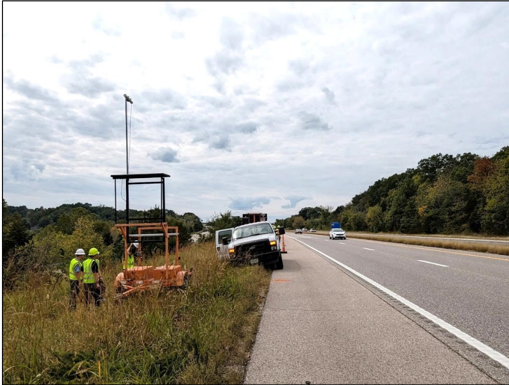
Figure 21. Roadside nonintrusive radar sensor
