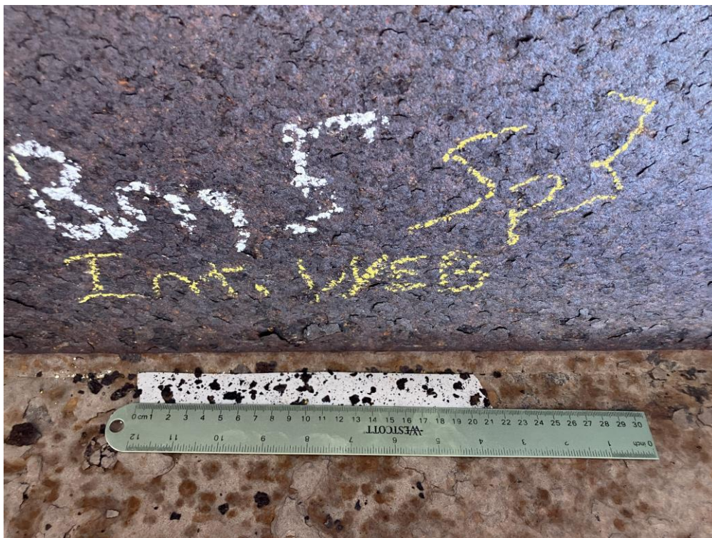
Figure 69. Photograph of a tape test conducted on the web of an interior beam belonging to No. 606750, dated December 12, 2023, from NBI inspection records.
