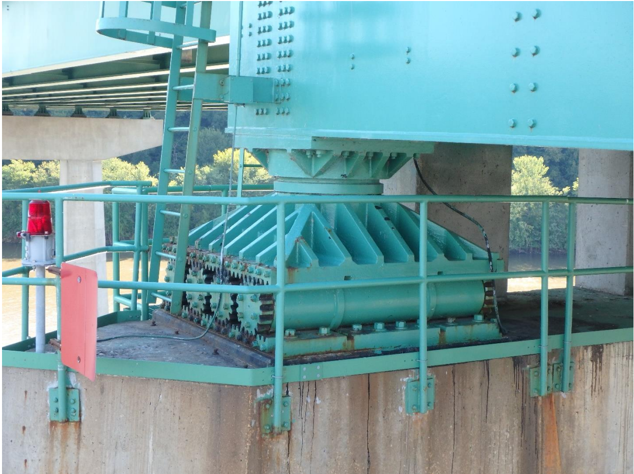
Figure 98. Roller bearing beneath tied-arch on US 61 over the Mississippi River
