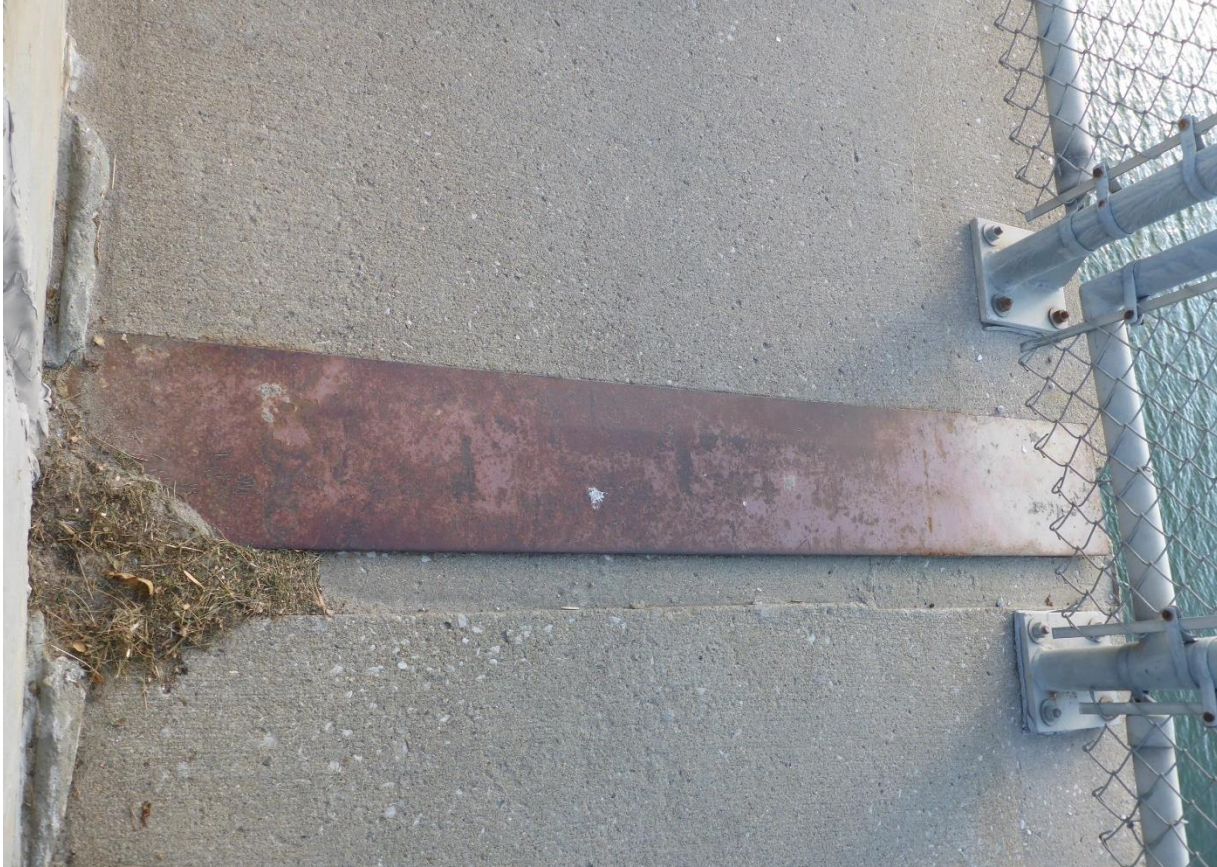
Figure 79. Sliding plate joint in sidewalk on Iowa 926 over the Des Moines River
