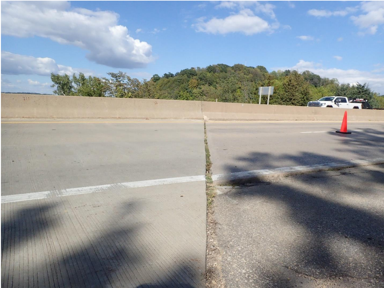
Figure 77. Pourable joint on US 62 over Mississippi River that has become an open joint
