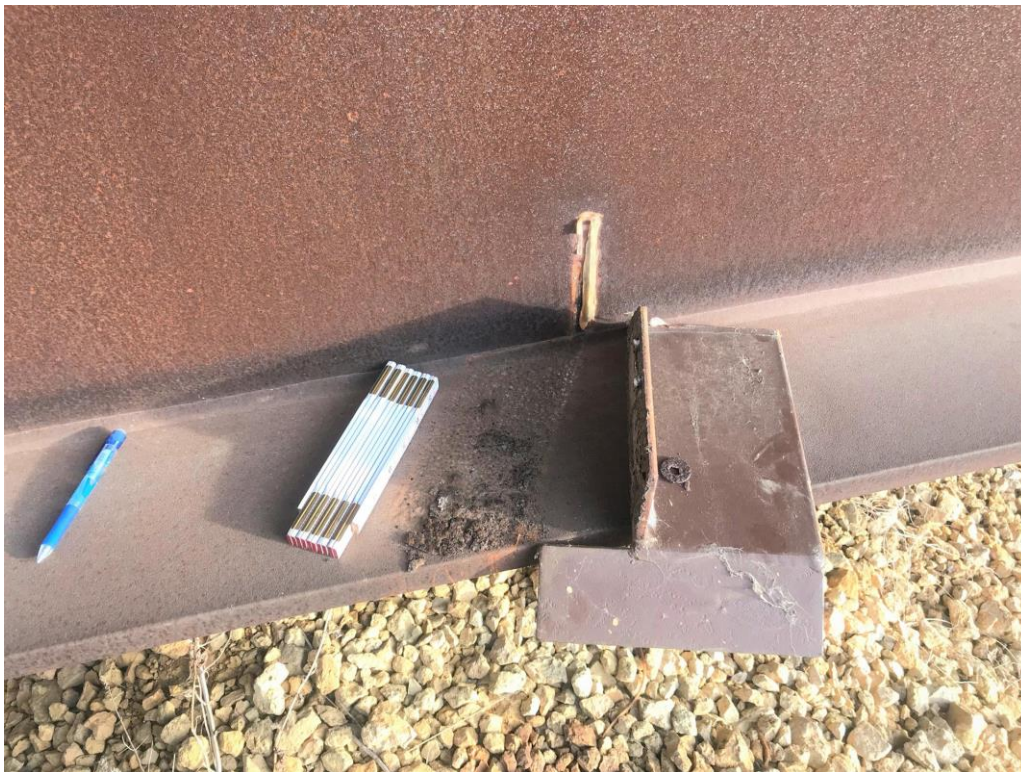
Figure 76. Photograph of a loose deflector plate on No. 606750, dated December 23, 2019, from NBI inspection records.
