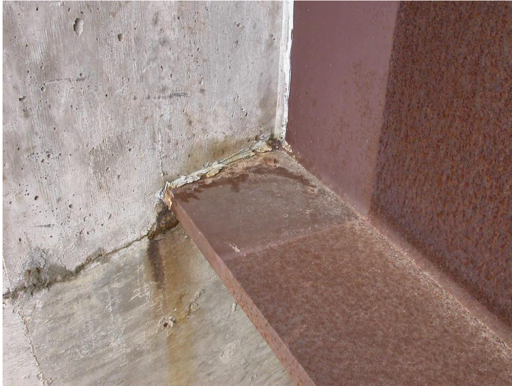
Figure 70. Photograph of rust products implying corrosion at an abutment belonging to No. 606750, dated May 6, 2015, from NBI inspection records.
