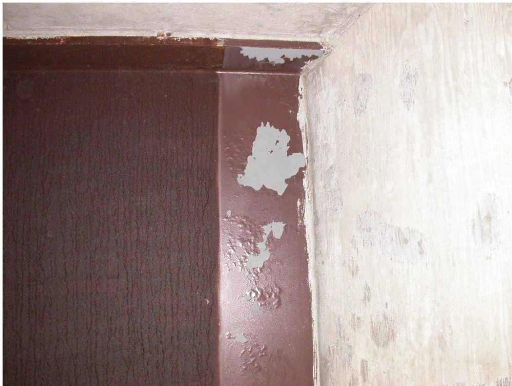
Figure 71. Photograph of peeling paint adjacent to an abutment belonging to No. 606750, dated May 6, 2015, from NBI inspection records.
