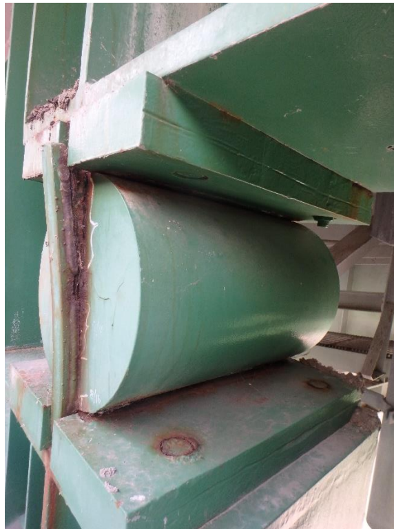
Figure 100. Pack rust and weld cracking at pintle bars in roller hinge bearings on I-80 Eastbound over the Missouri River
