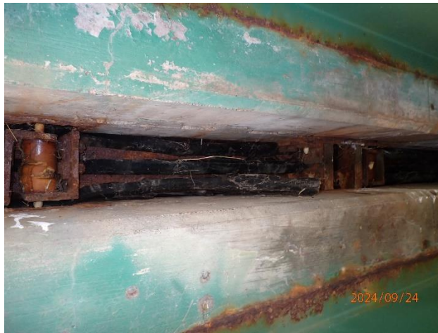
Figure 85. Underside of modular joint
