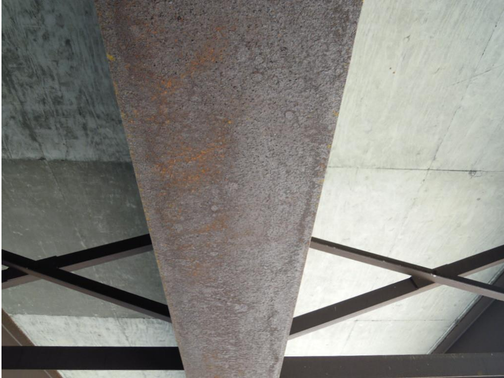
Figure 73. Photograph of typical “light flaking rust above roadways” on underside of a bottom flange of a girder belonging to No. 609280, dated September 29, 2010, from NBI inspection records.
