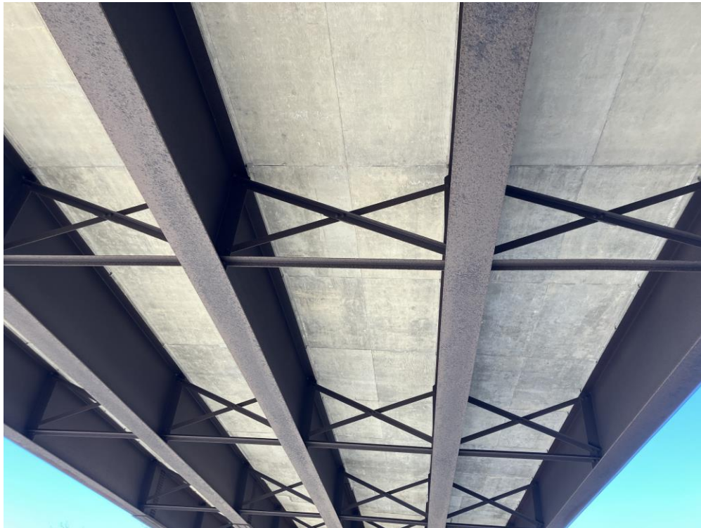
Figure 68. Photograph of the typical appearance of the floor system of No. 606750, dated December 12, 2023, from NBI inspection records.
