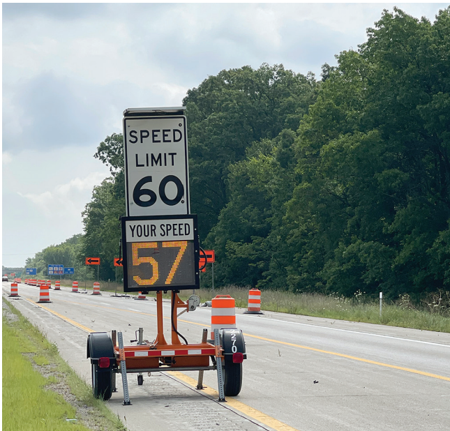
Speed feedback trailer in a freeway work zone lane closure in Michigan
