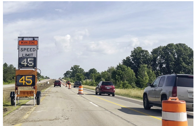
SFT + DSL assembly deployed in a freeway lane closure in Michigan
