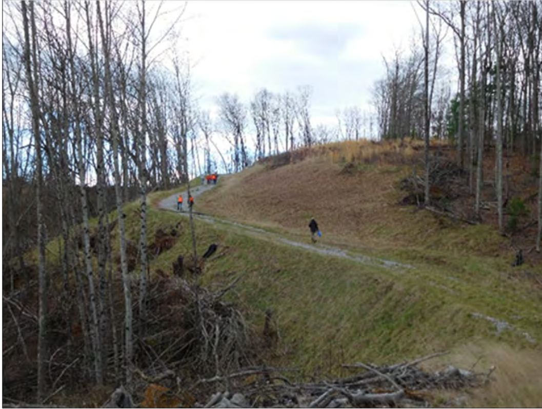
FIGURE 8 Permanent forest access road that was planned and laid out by students taking the Forest Boundaries and Roads course.
