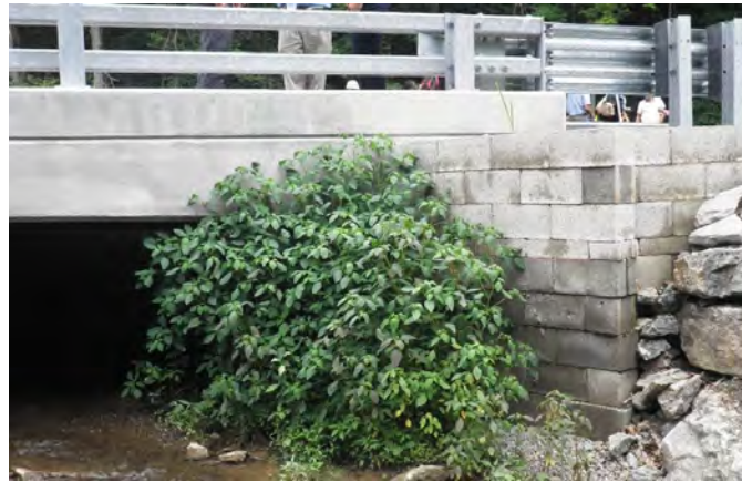
FIGURE 1 A GRS bridge abutment constructed in Pennsylvania using modular concrete blocks for the abutment facing.
