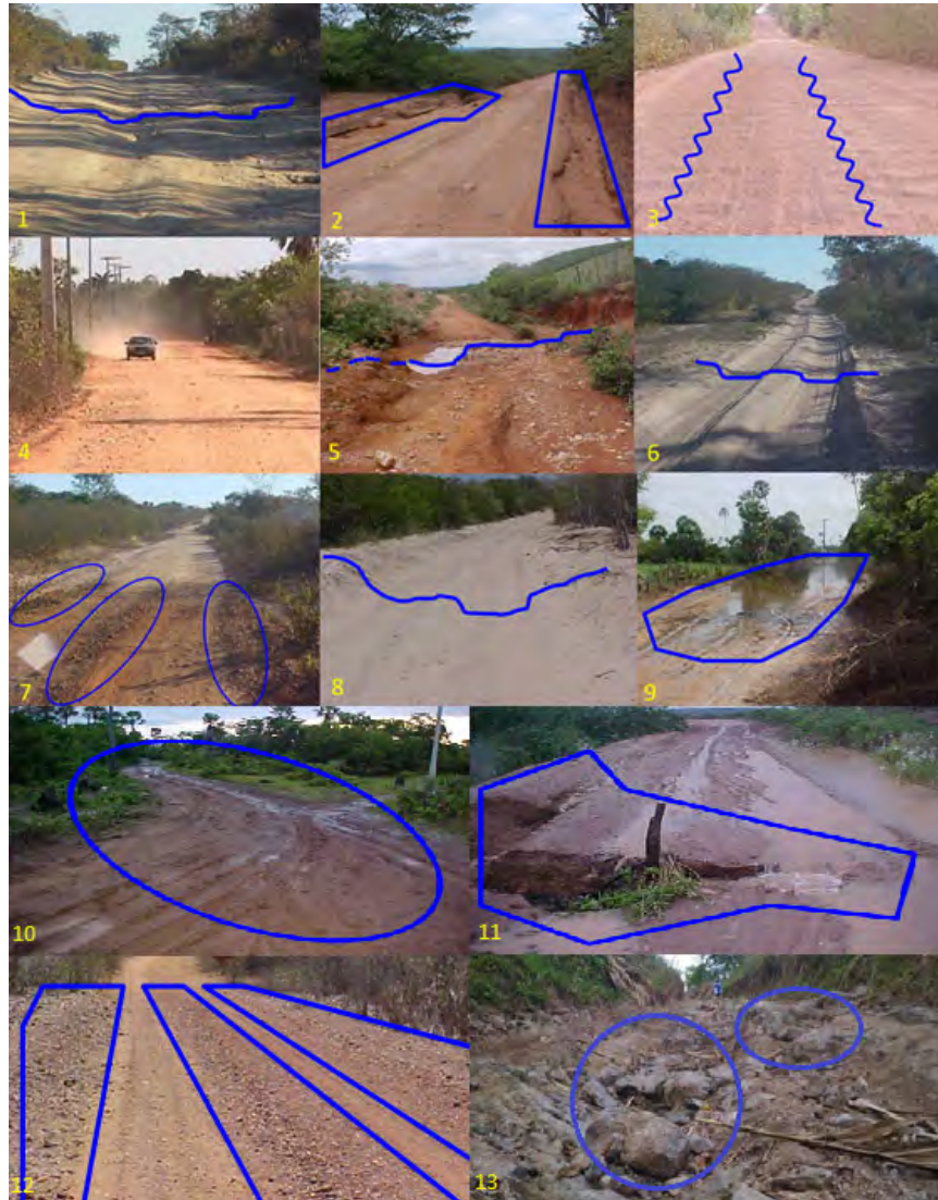
FIGURE 3 Examples of pavement defects.
