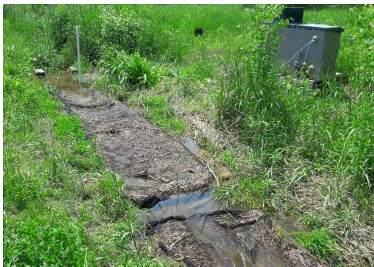
FIGURE 1 Woodchip bioreactor sock installed in ditch with ISCO sampler housing and rain gage in the background.
