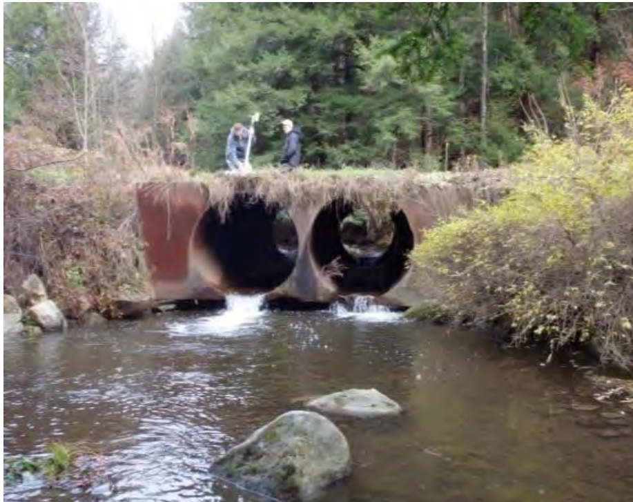
FIGURE 1 Before: twin 7-ft “tanker car pipes” bankfull-width channel created a barrier in a reproducing brook trout stream, and because it often clogged, flooded the road and required maintenance. (Photo: Tioga County Conservation District.)
