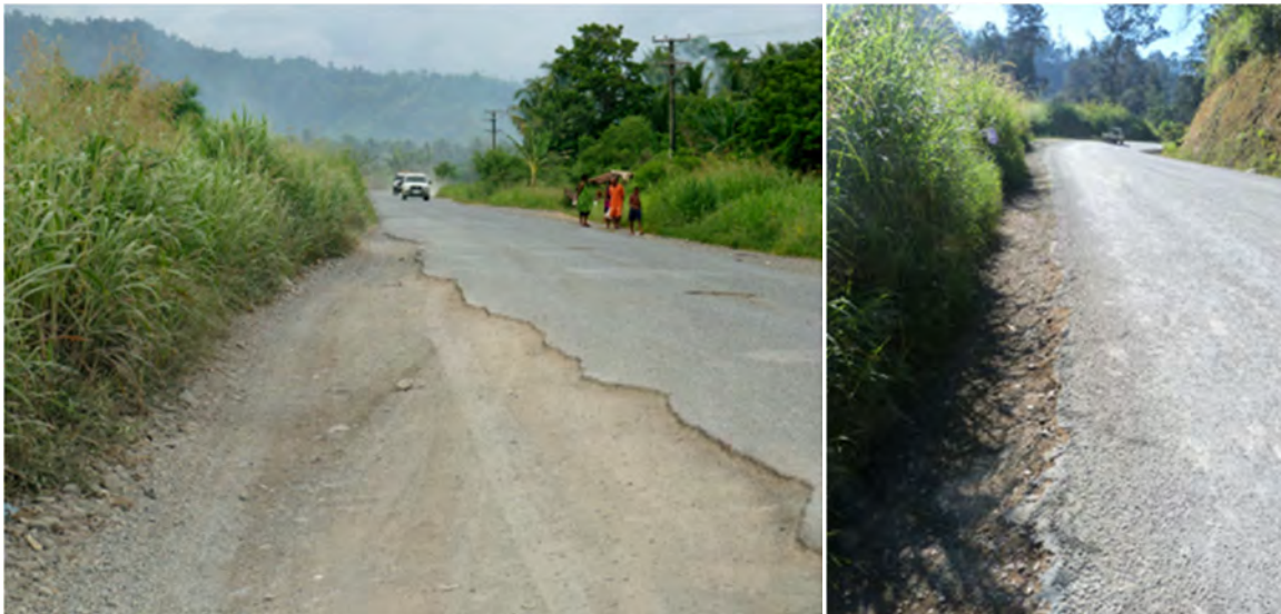
FIGURE 2 Distresses were more prevalent where poor drainage was encountered. Vegetated growth was the principal contributor to poor drainage.
