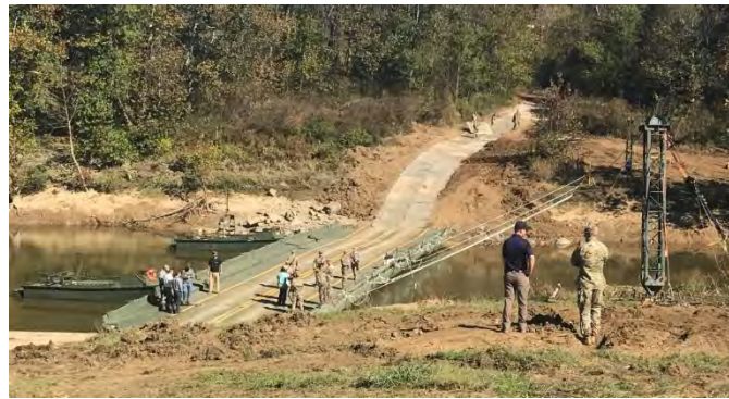
FIGURE 6 A 96-ft-long section of ACE Mat being placed on a horizontally and vertically curved route up a river bank.
