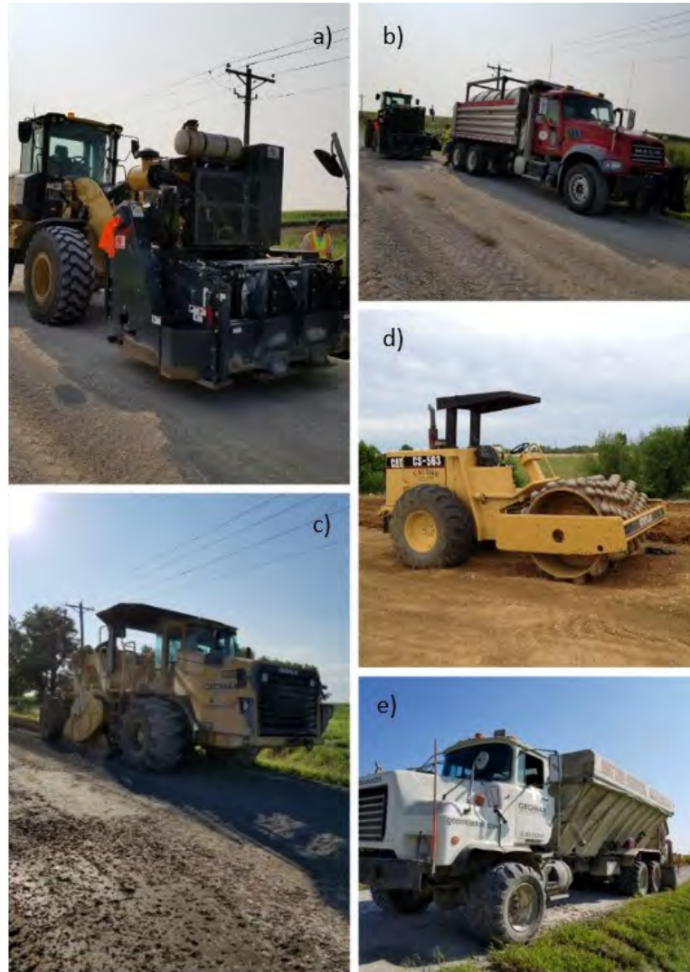
FIGURE 2 Equipment used for chemically stabilized sections: (a) RoadHog reclaimer; (b) water truck with chemical stabilizer added to tank connected to RoadHog; (c) road reclaimer; (d) sheepfoot vibratory compactor; and (e) powder spreader truck.
