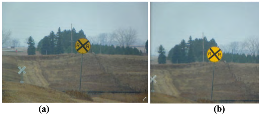
FIGURE 2 (a) Before and (b) after LED illumination photos, taken to develop a sign condition rating.
