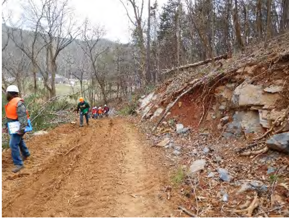
FIGURE 1 Students examine the template for a newly installed forest log truck access road.
