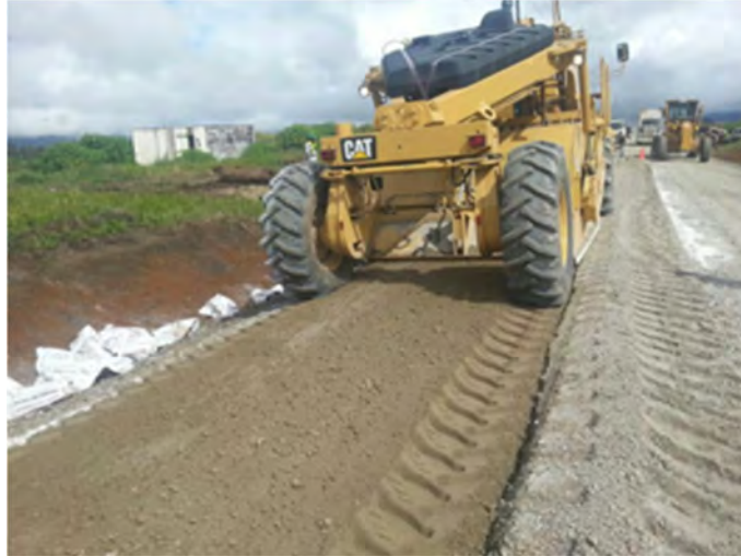
FIGURE 3 A soil recycler was used to blend the various materials and layer thicknesses, to help break down some of the rounded nature of the alluvial stones that had been used in the original pavement design, as well as to achieve a homogenous mix, stabilizer distribution, and optimum moisture content (OMC).
