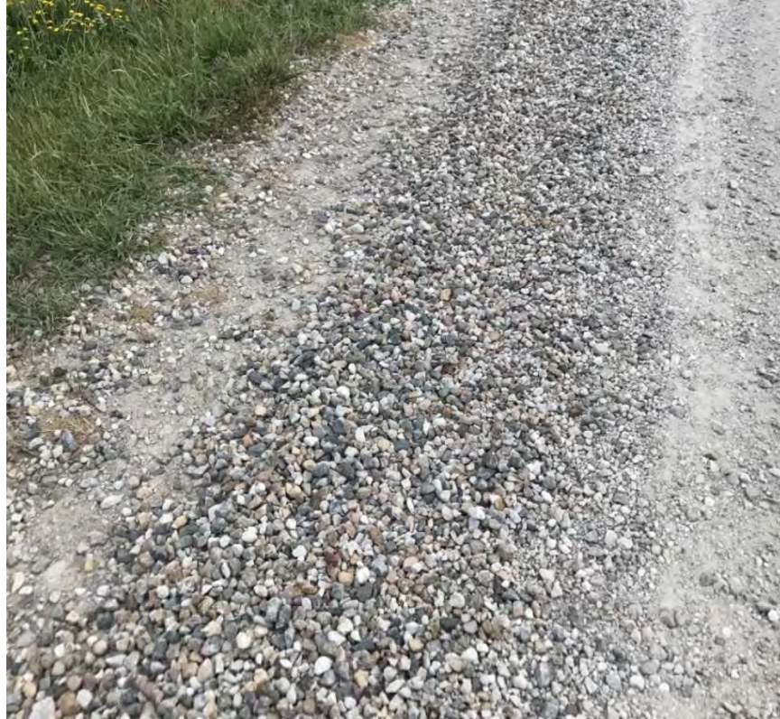
FIGURE 8 Movement of the loose aggregate materials to the sides of the road for Section 7 (70%BFL Class A + 30% CRG clean).
