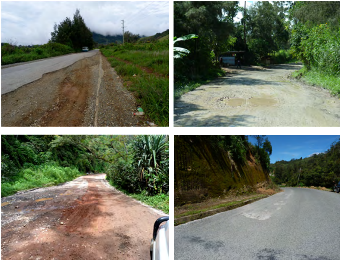
FIGURE 1 Distresses observed during the pavement investigation included stripping of the wearing course, edge-break, and potholing in both the sealed and exposed pavement.
