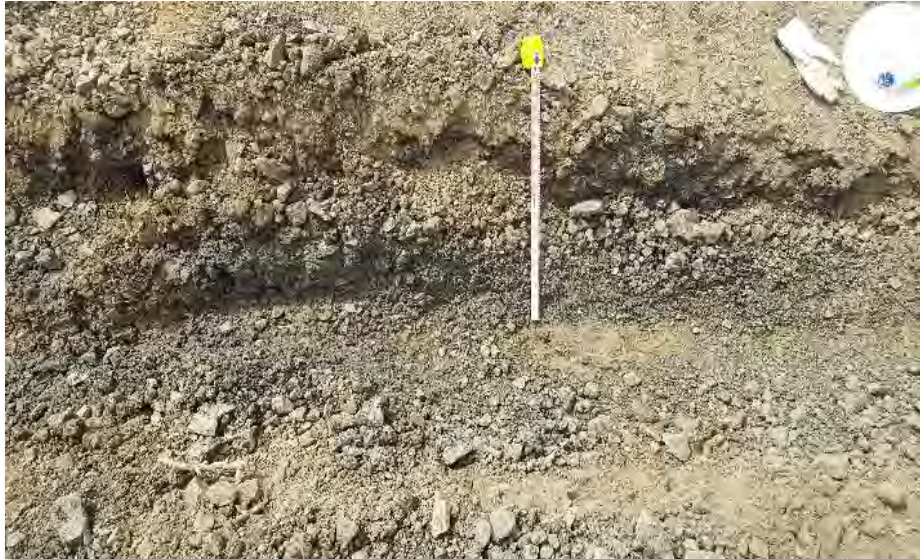
FIGURE 3 Outside heaving of the geogrid treatment.
