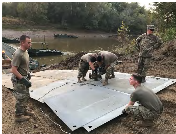
FIGURE 7 Army soldiers placing the fiberglass mat up a riverbank using only an electric impact wrench.
