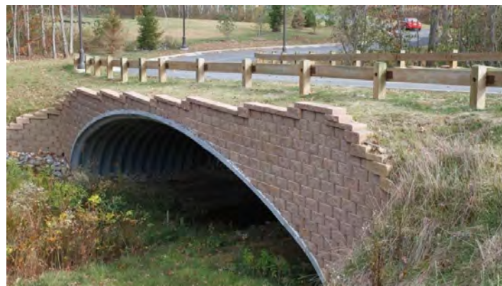
FIGURE 2 A CMP-buried bridge with a 56-ft span built on a rural road (photo courtesy of Joel Hahm).
