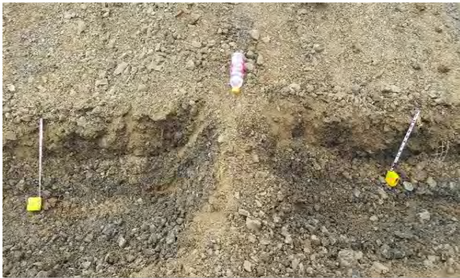
FIGURE 4 Heaving and rupture of the geofabric section.
