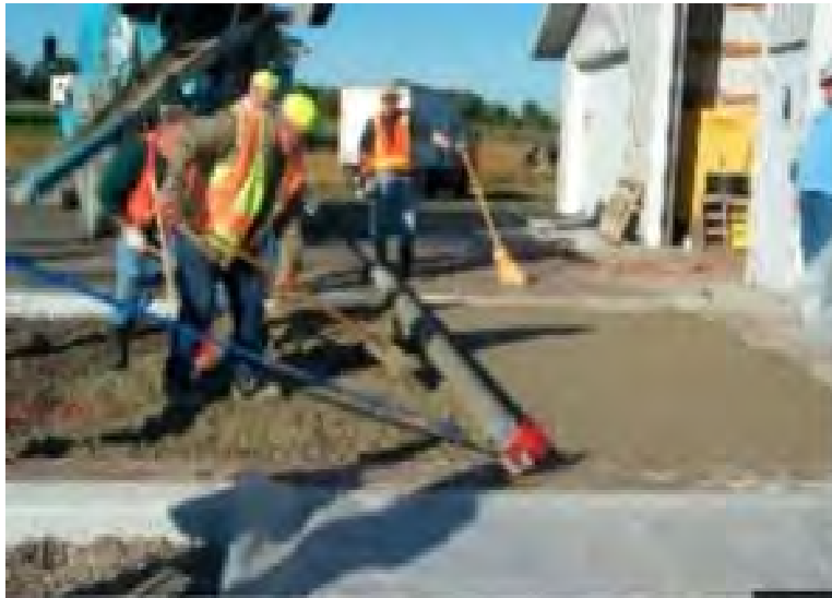
FIGURE 1 MnROAD pervious concrete driveway: placement and motorized screed compaction of pervious driveway.
