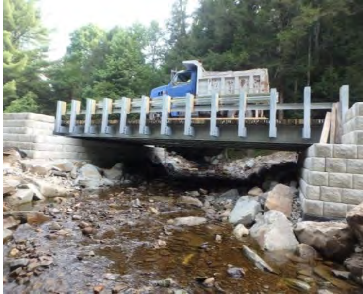
FIGURE 2 After: 32-ft geosynthetically in a 30-ft reinforced soil bridge used to span bankfull in a channel width. (Photo: Tioga County Conservation District.)
