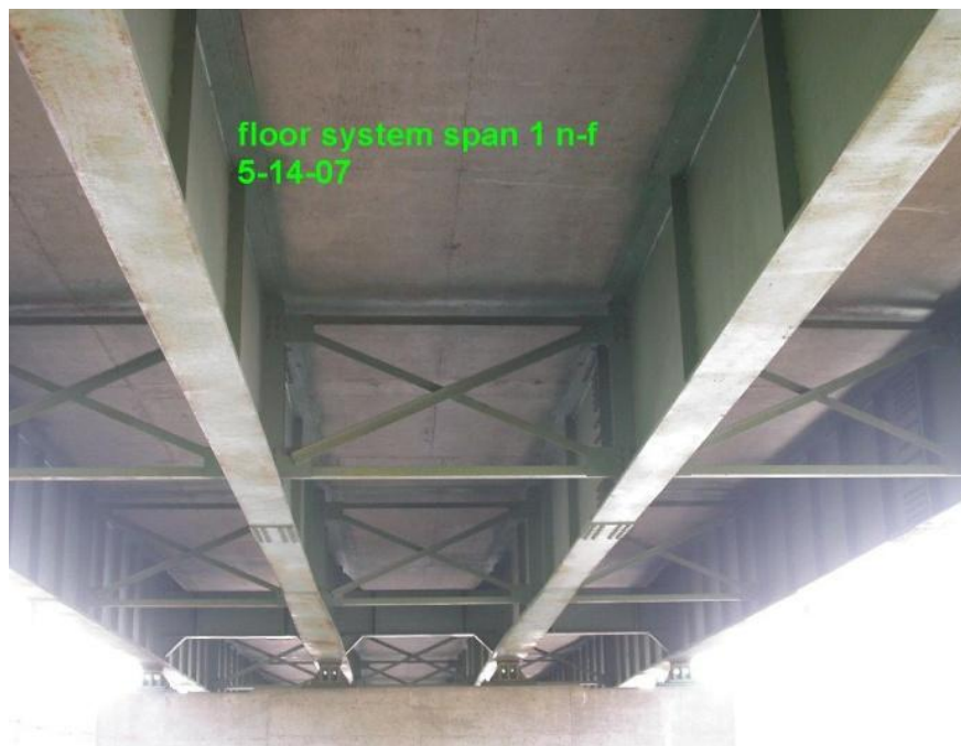
Figure 3. View of underside of bridge. Note the channel diaphragms at the pier.
