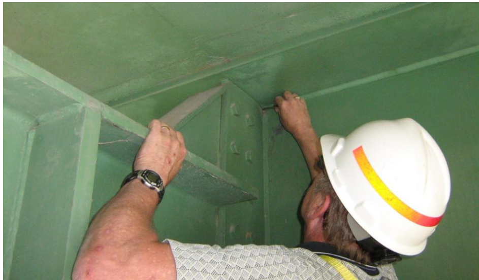
Figure 8. Inspection and measurement (with feeler gage) of pier bearing stiffener fit with top flange of girder.
