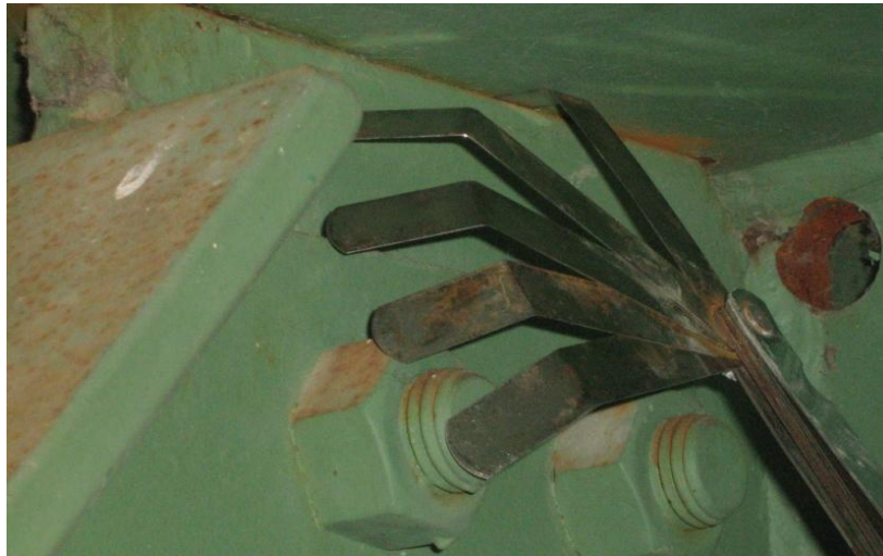
Figure 20. Feeler gage inserted between top of bearing stiffener and Girder 4 top flange at Pier 6. Note the corrosion between the interfaces and also note the retrofit hole that had been previously drilled to arrest a fatigue crack in the girder web.
