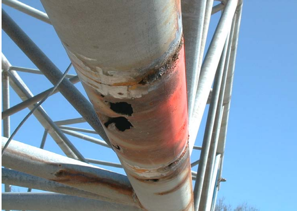
Figure 2. Deterioration of Bottom Chord Member of the Truss
