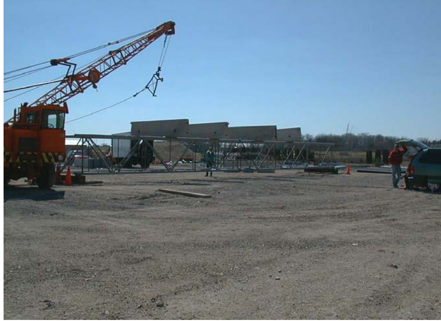
Figure 6: Sign Truss Loaded with Four Concrete Blocks
