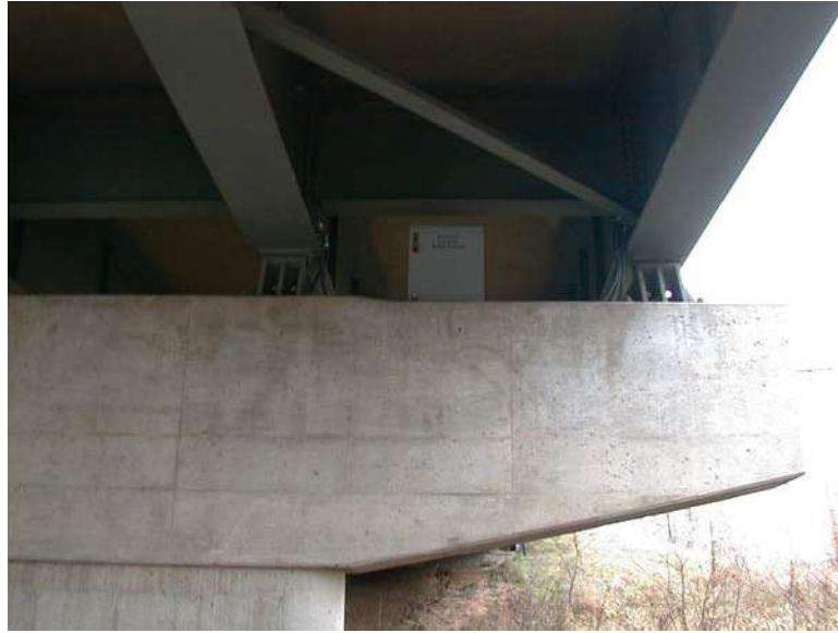
Figure 4.9. Photograph of DAS enclosure on Pier 2.
