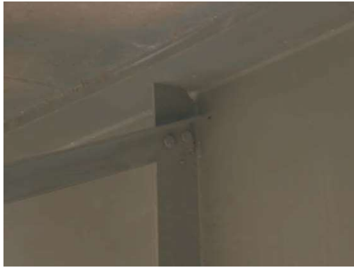
Figure 4.6. Photograph of typical web gap.
