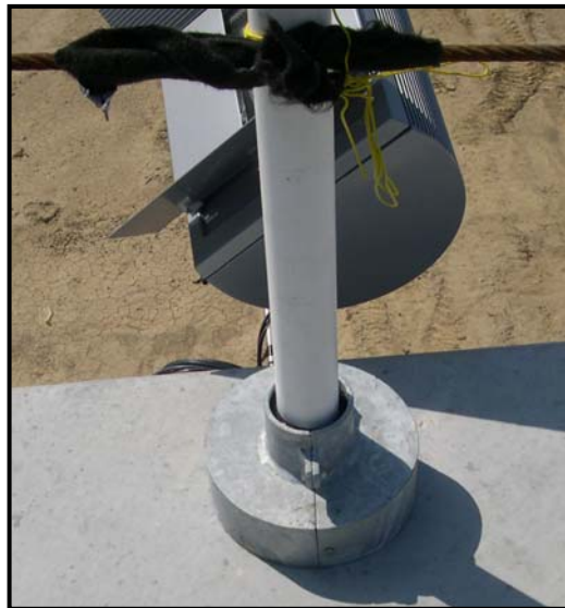
Figure 5. Galvanized trumpet pipe cover provides UV protection for FBG sensors leads
