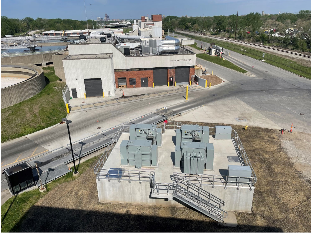
Figure 2: Elevated Electrical Transformers the Serve Main Pump Building and floodwall protecting Preliminary Treatment Building in background
