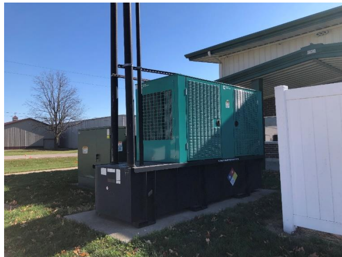
Backup generator, providing power to the water treatment plant or wells in the event of a power outage
