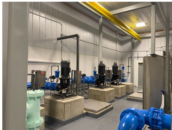
High service pumps to distribution system
