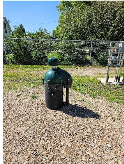
New well, not yet in service
