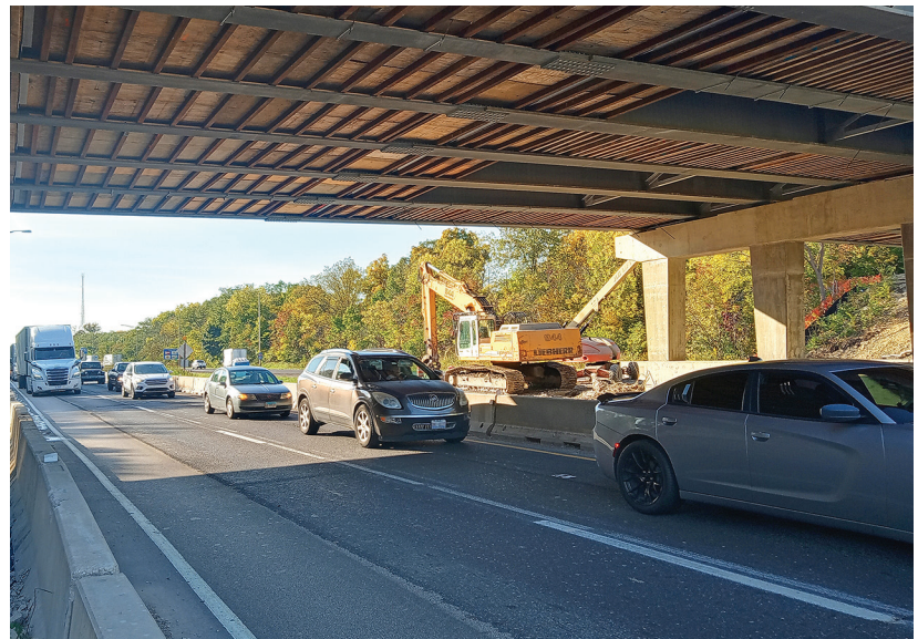
Vehicles passing through a work zone with two open lanes bounded by concrete barriers
