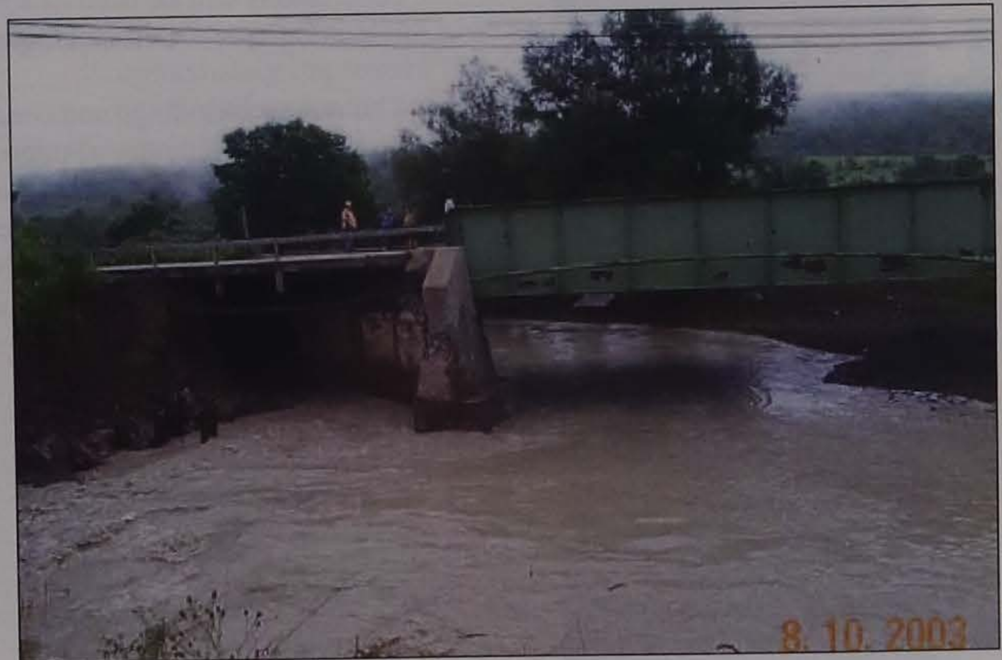
Waterway scour threatens bridge abutment and embankment.
