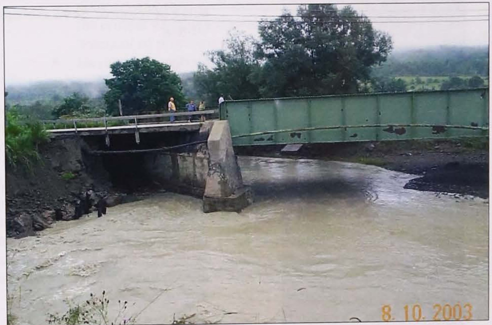
Waterway scour threatens bridge abutment and embankment.
