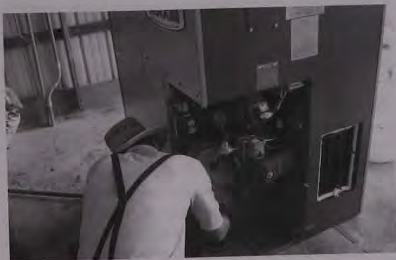
Figure 3. Installation of a biomass boiler cost-shared by the Local Bioenergy Initiative.
