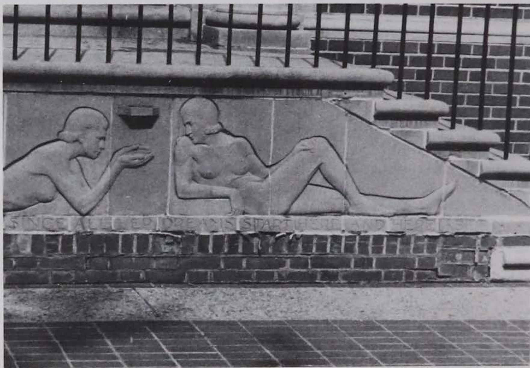
DETERIORATION OF TERRA COTTA AND MASONRY MORTAR JOINTS OF ROBERTS HALL FOUNTAIN, 1983. AUTH
