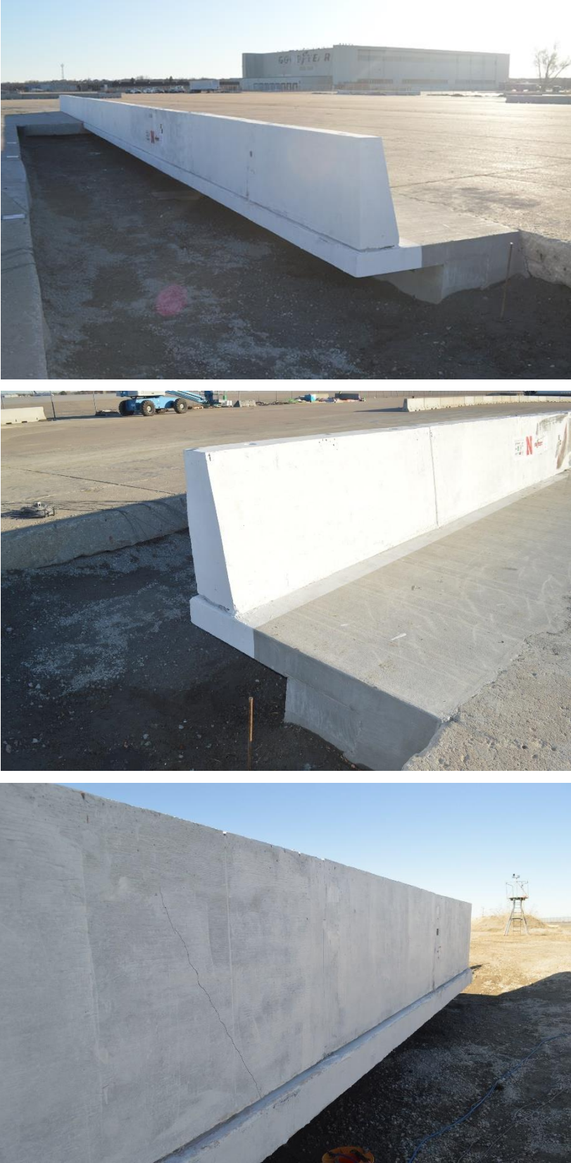
Figure 93. Deck Damage, Test No. ABCBRM-1
