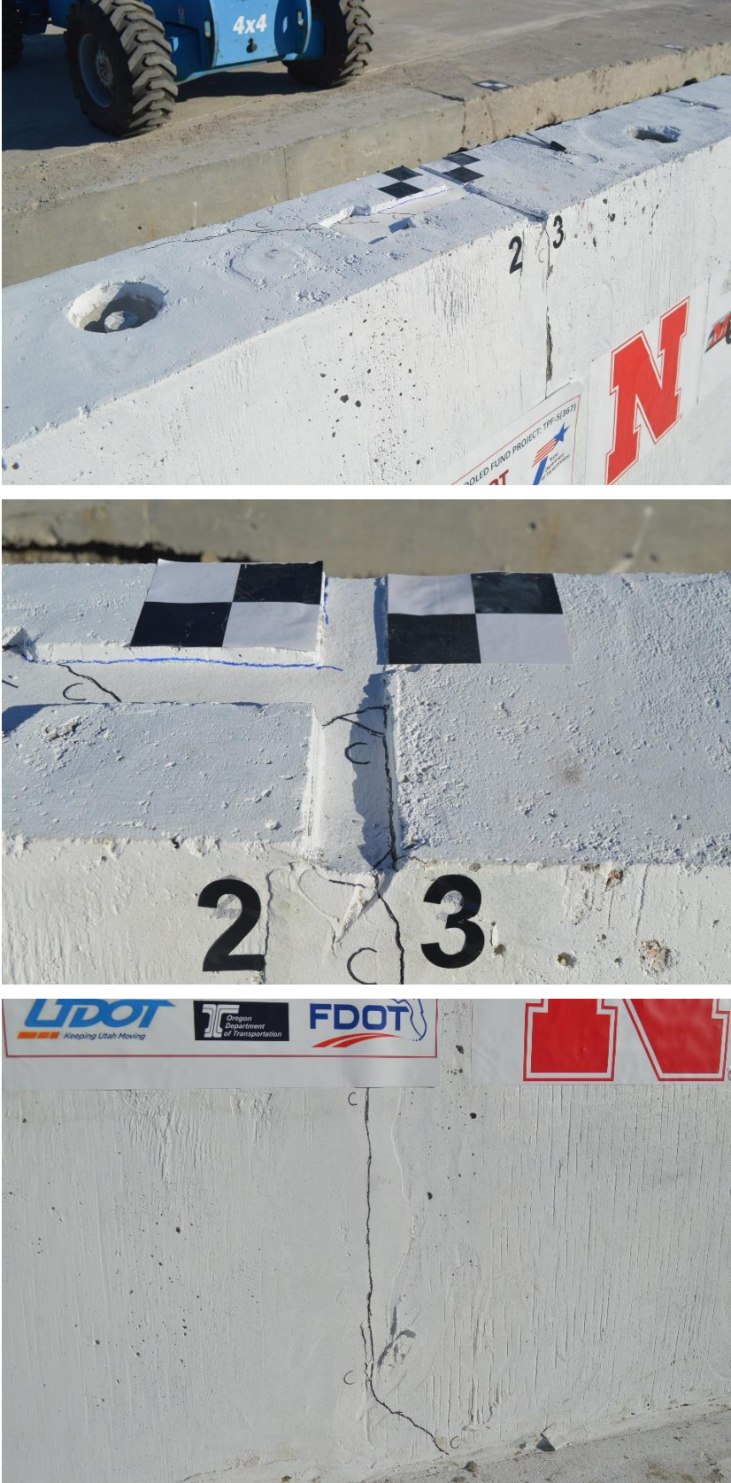
Figure 91. System Damage, Barrier Segment Nos. 2 and 3, Test No. ABCBRM-1
