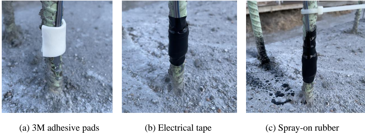
Figure 79. Strain Gauge Protection System
