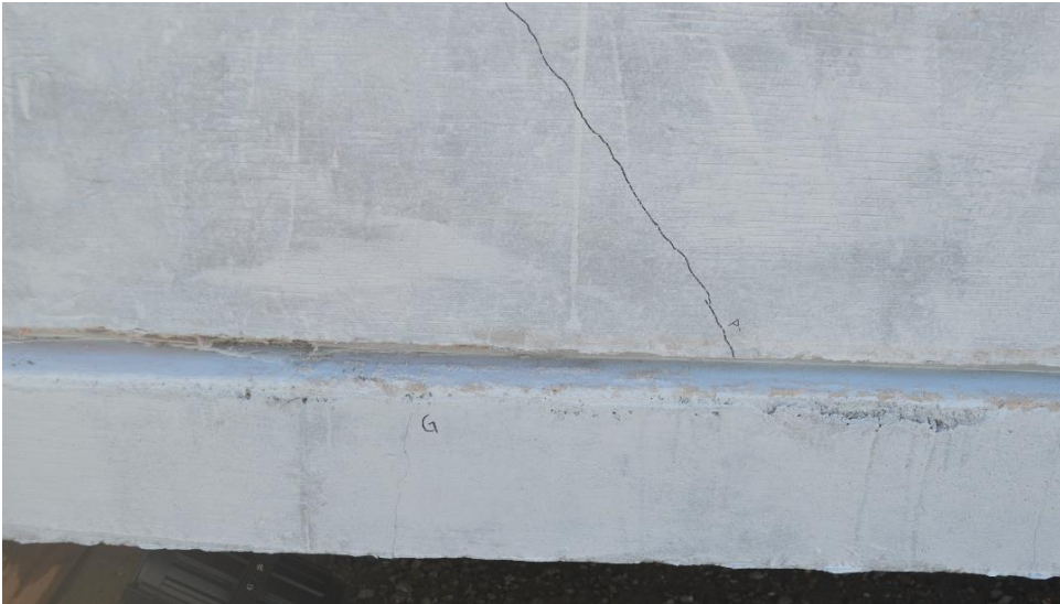
Figure 92. System Damage, Backside of Bridge Rail, Test No. ABCBRM-1
