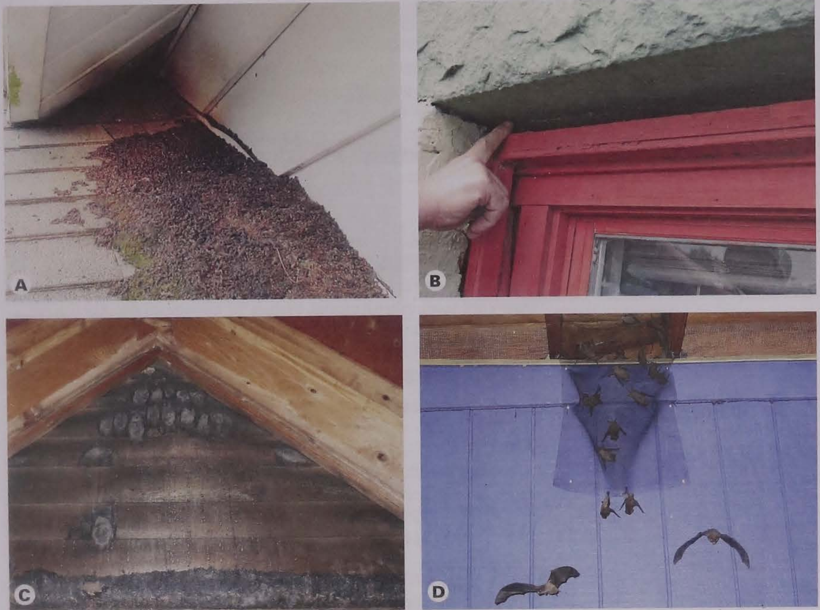
Figure 12.5. (A) Bat entry under roof overhang, note accumulated excrement; (B) Bat entry above window; (C) Bat roost at attic end vent; (D) Bat exclusion device. Image credit: (A) Matthew Grady, www.batguys.com ; (B) Verron Federation, http://animaltrappingremoval.com/batremoval/ ; (C) http://dnfreetime.com ; (D) www.aaanimalcontrol.com
