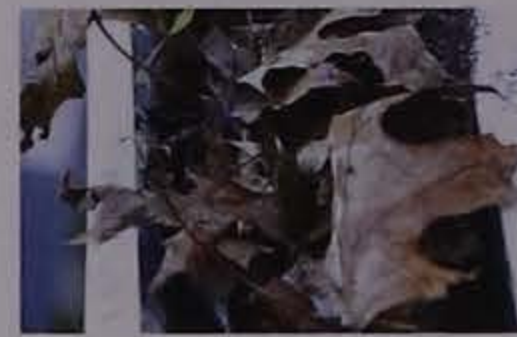
Clogged roof gutter, a mosquito breeding site. M.H. Shour, Iowa State University Extension
