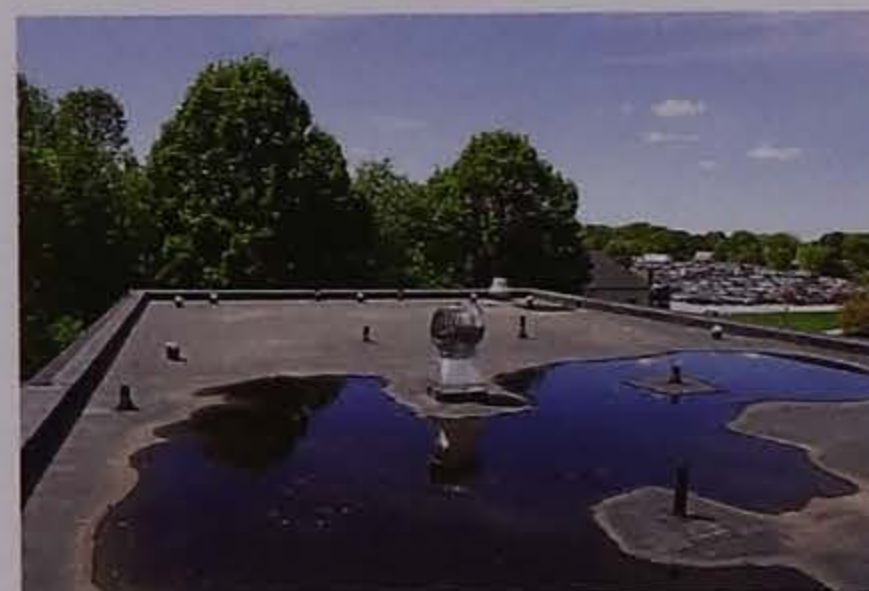
Figure 3.7. Rainwater standing on flat-roofed building. Photo credit: M.H. Shour, Iowa State University Extension
