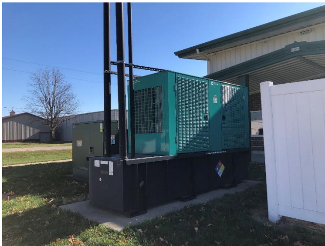
Backup generator, providing power to the water treatment plant or wells in the event of a power outage
