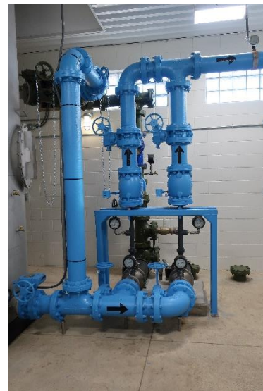
Water treatment plant pumps
