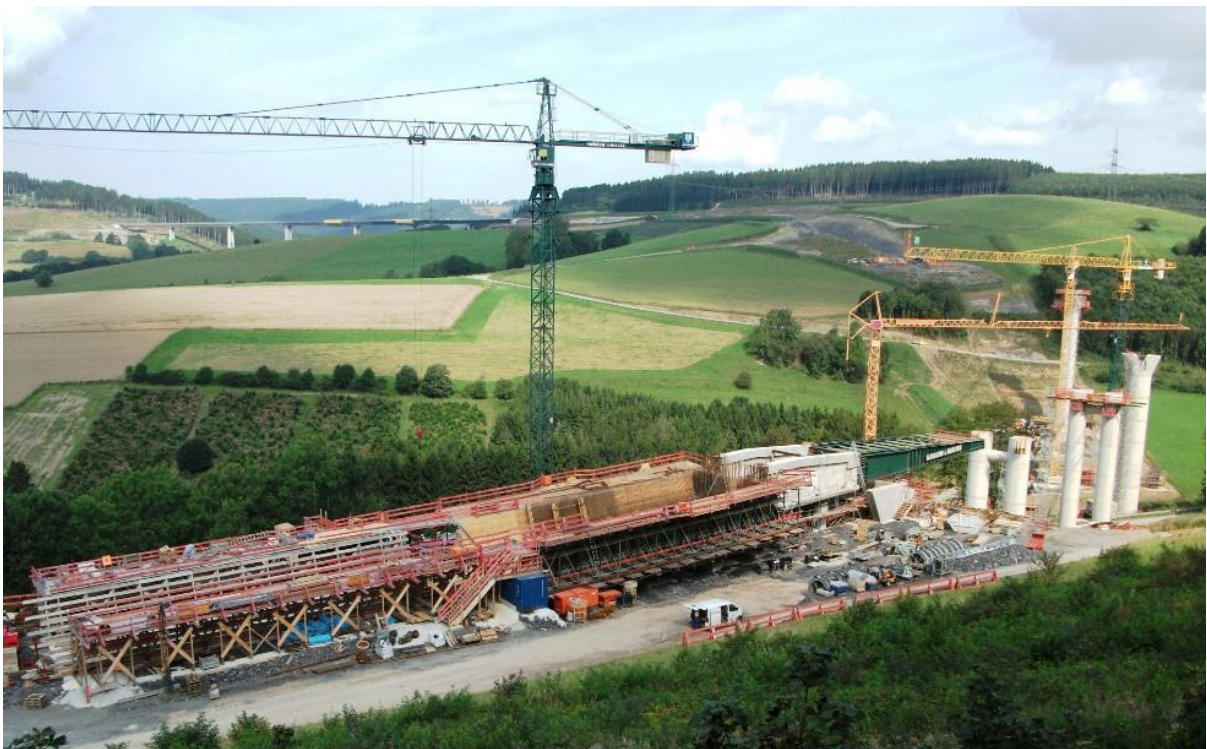
Figure 61 Example of a casting bed
