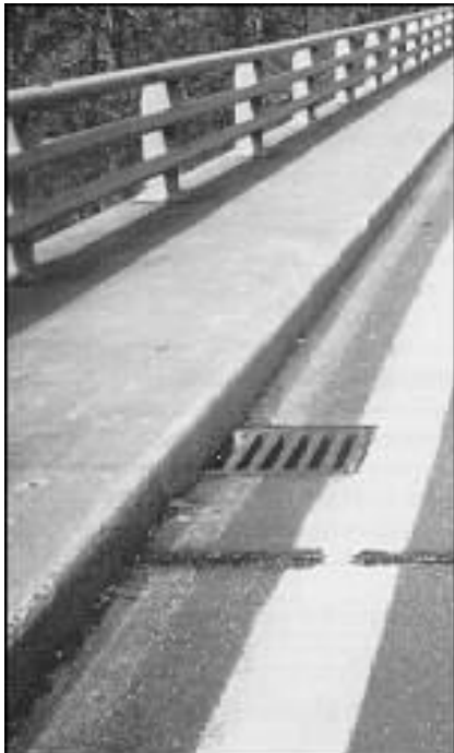
Figure 55 Example of pipes on a bridge
