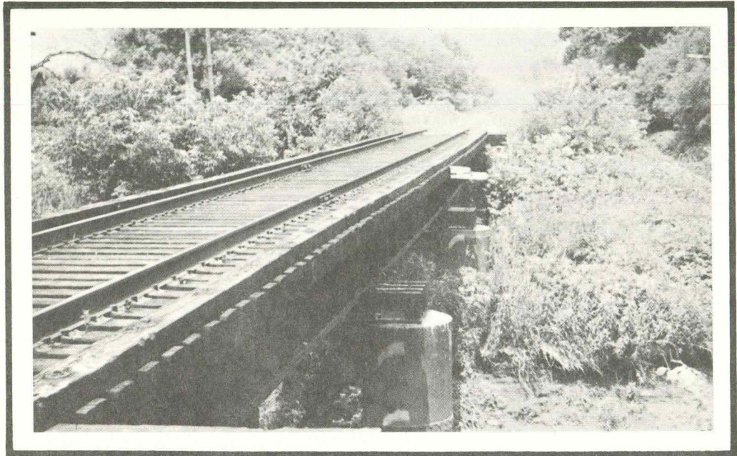
Figure 9. Downstream side of C.R.I.&P. RR bridge at mile 9.62 (West Branch), looking north.
