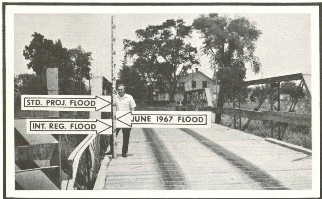
Figure 32. Upstream side of County Road bridge at mile 9.97 (West Branch), looking north.
