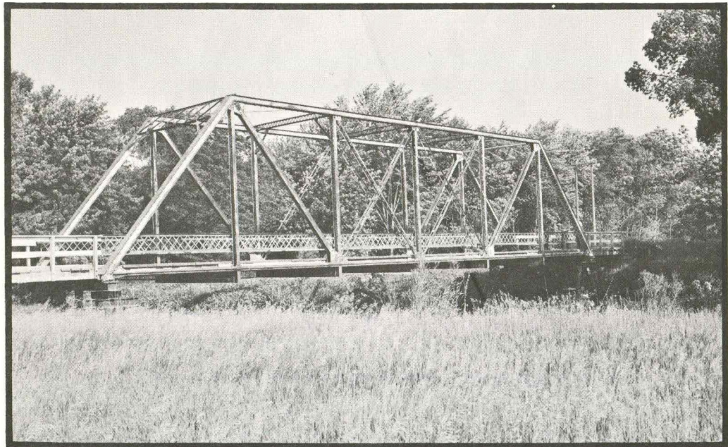
Figure 18. Downstream side of the Main Channel bridge on West County line road at Mile 14.57.
