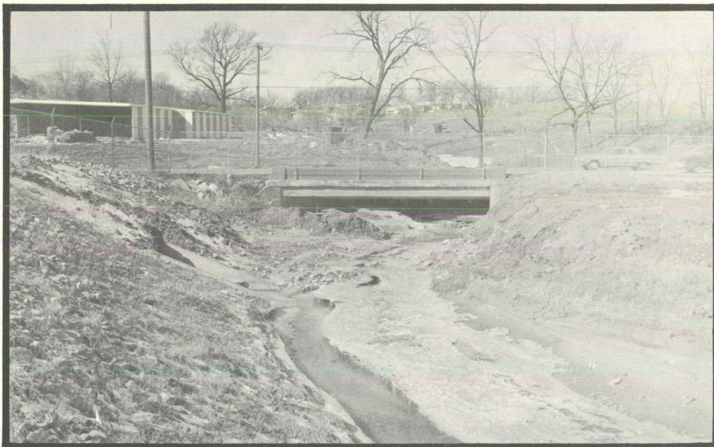
Figure 16. Looking upstream at the Isett Avenue bridge over Mad Creek at Muscatine, Iowa.
