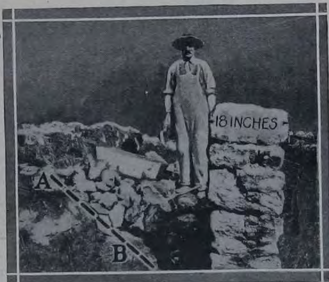
FIG. 2.—Unsatisfactory Cellar Wall.
