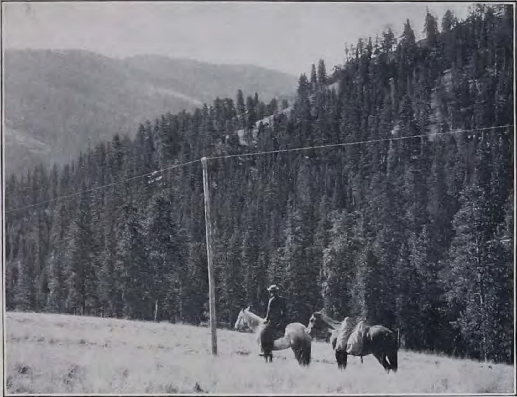
FIG. 1.—A TELEPHONE LINE IN THE WALLOWA NATIONAL FOREST, OREGON.
