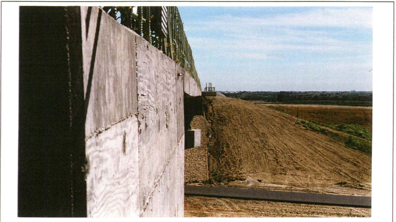
Figure 11 View of bridge abutment and slab end showing formwork joint leaks and variable depth of slab resulting in a “fishbelly” effect.
