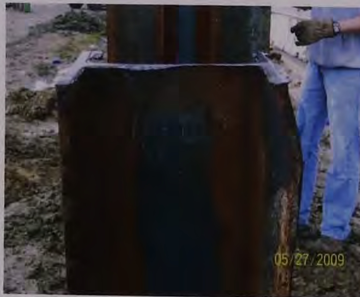
Figure 4.16. Minimal buckling on flanges at pile head
