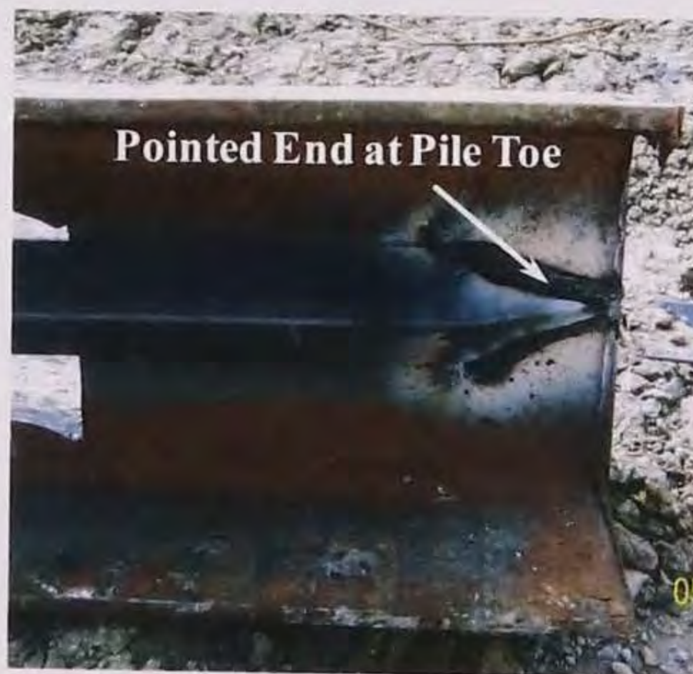
Figure 4.5. Angle bars were chamfered to form a pointed end at pile toe
