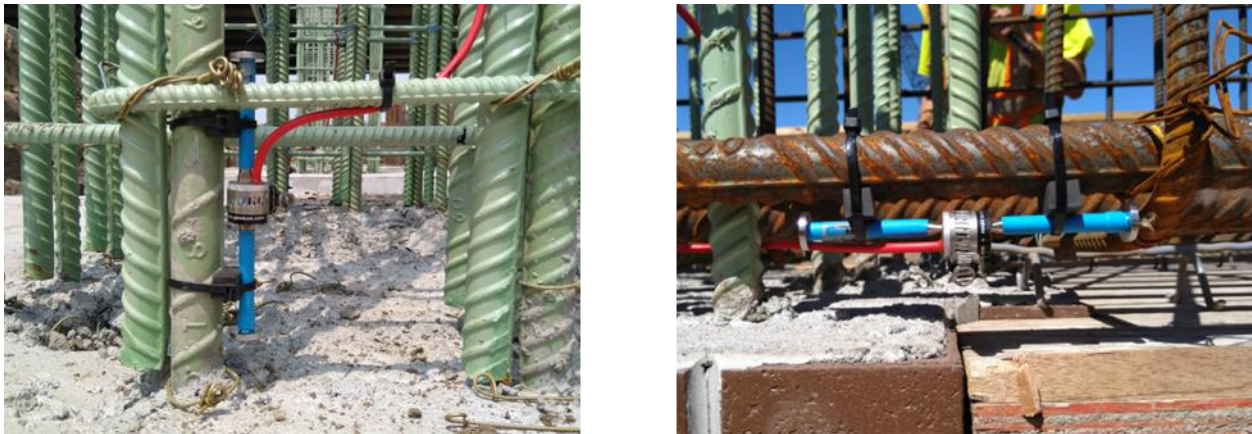
Figure 3.10. 418 Woodbury bridge sensor placement at column base (left) and cap beam (right)
