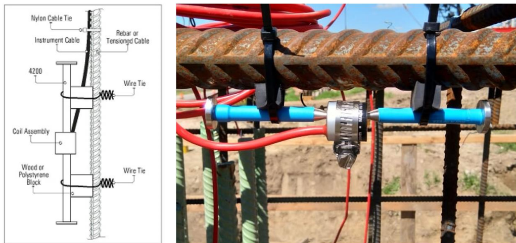
Figure 3.4. Sensor installation as recommended by manufacturer (left) and as installed in the field (right)
