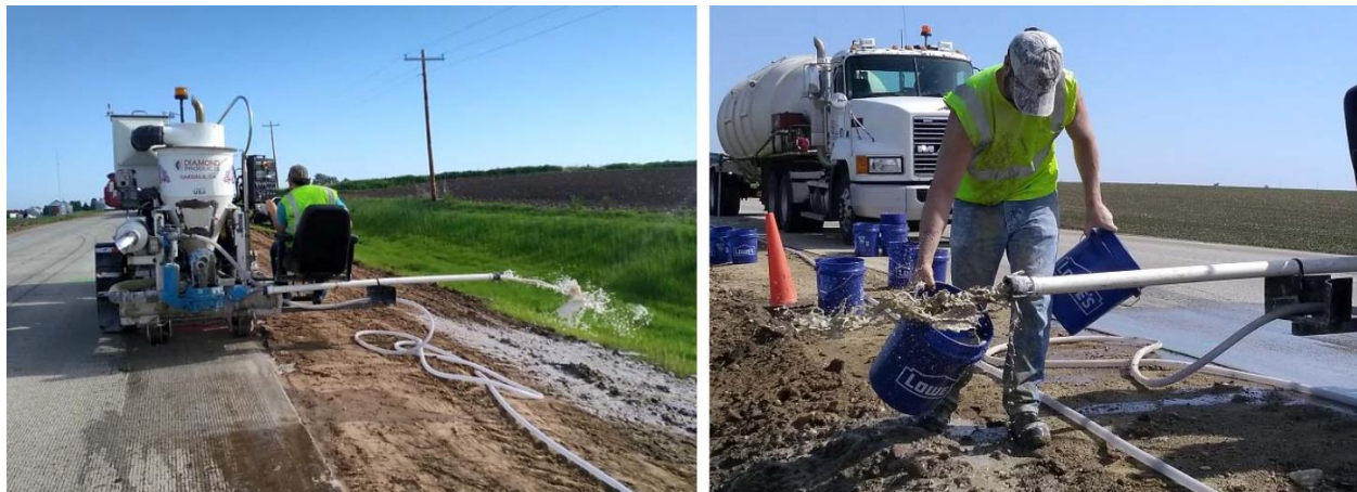
Figure 2. Direct discharge CGR collection (site CGR-3)
