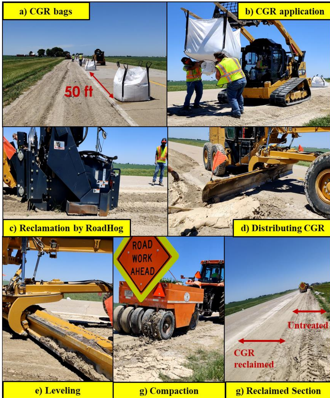
Figure 52. Construction of CGR Reclaimed section in Washington County: (a) placing CGR bags at the designated distance, (b) dumping CGR, (c) reclaiming soil with CGR using a RoadHog, (d) distributing CGR by blading, (e) leveling the surface, (f) compaction, and (g) completed CGR Reclaimed section
