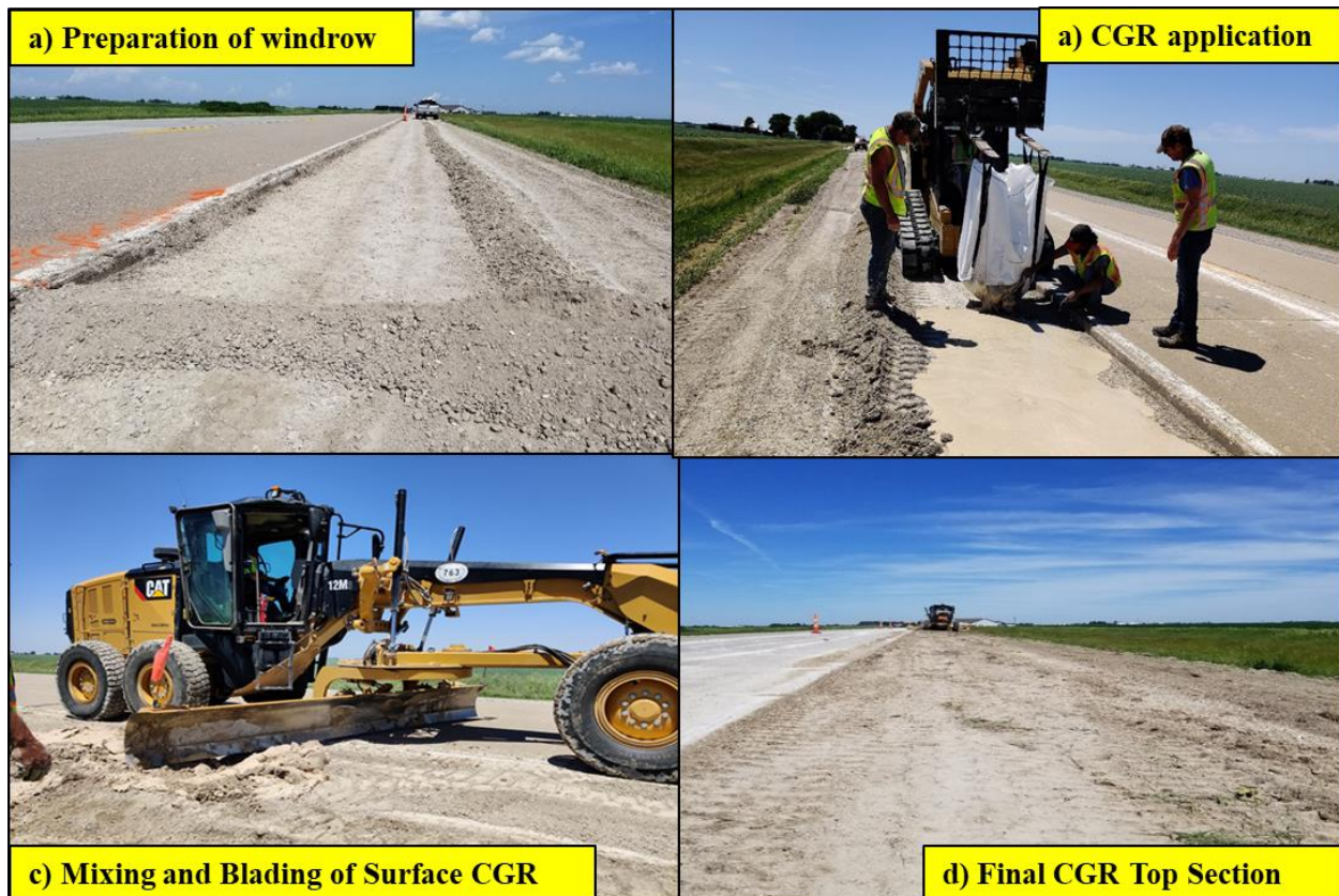
Figure 53. Construction of CGR Top section in Washington County: (a) creating windrow, (b) dumping CGR, (c) mixing and blading CGR, and (d) completed CGR Top section
