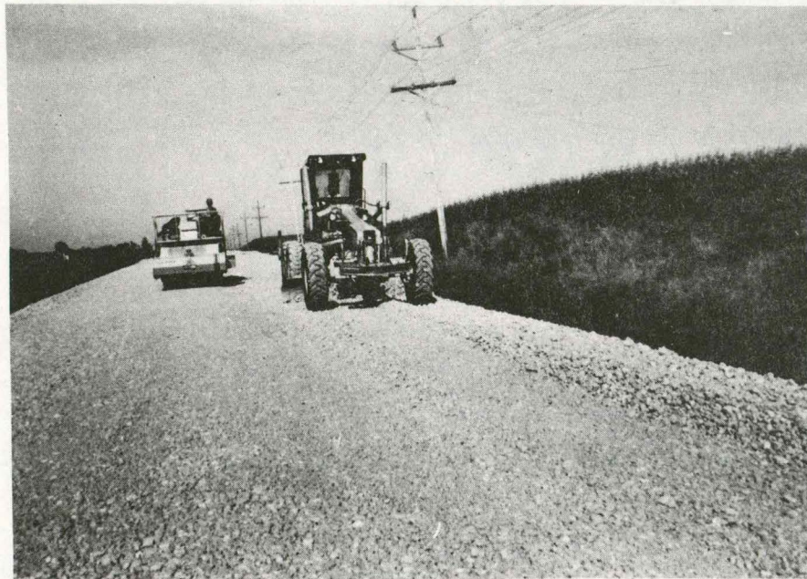
Motor grader working the excess macadam. This is not the recommended procedure since it causes segregation of the stone.
