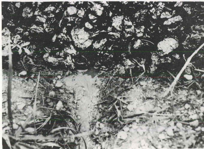
3" emulsion bound macadam base showing water running to the ditch.
