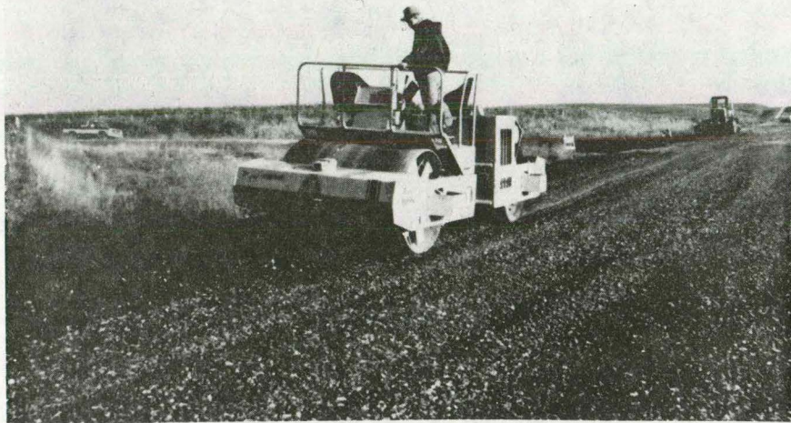
Vibratory roller passing over the emulsion bound macadam. The roller had a tendency to break the larger rock at the surface.
