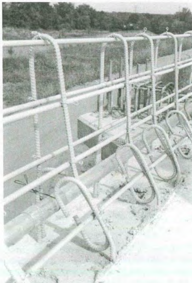
Figure 1: Conduit is run through one or both bridge rails so utility cables may be run through the bridge.
