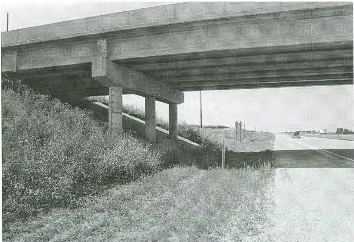
Figure 1: Side piers at newly-constructed four-span bridges require special grading, but no barrier.
