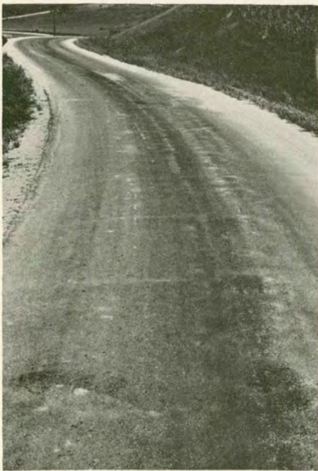
i. Surface condition of section N-2, August 25, 1980.
