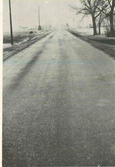
f. Surface condition of section HC-1, December 29, 1980.
