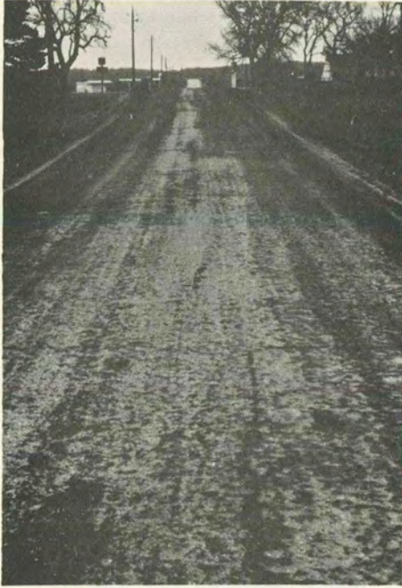
e. Surface condition of section HC-1, February 28, 1980.
