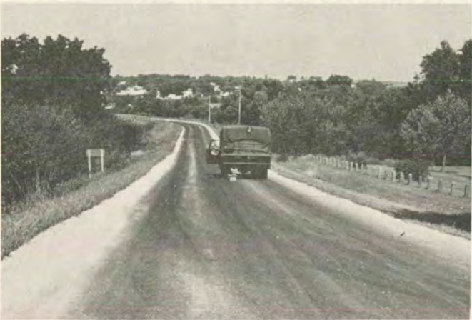
d. Surface condition of section N-1, August 25, 1980.
