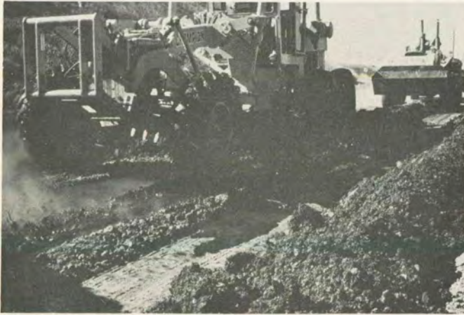
a. Asphalt emulsion application (left), initial fold over and longitudinal mixing (center), rotary mixer (rear), section N-1.
