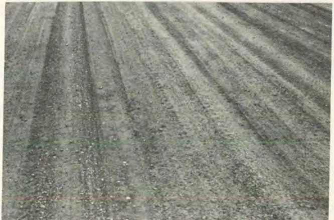
d. Surface condition immediately after spraying, August 28, 1980.
