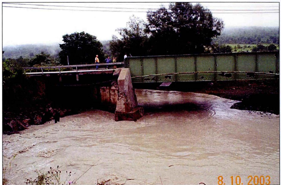
Waterway scour threatens bridge abutment and embankment.
