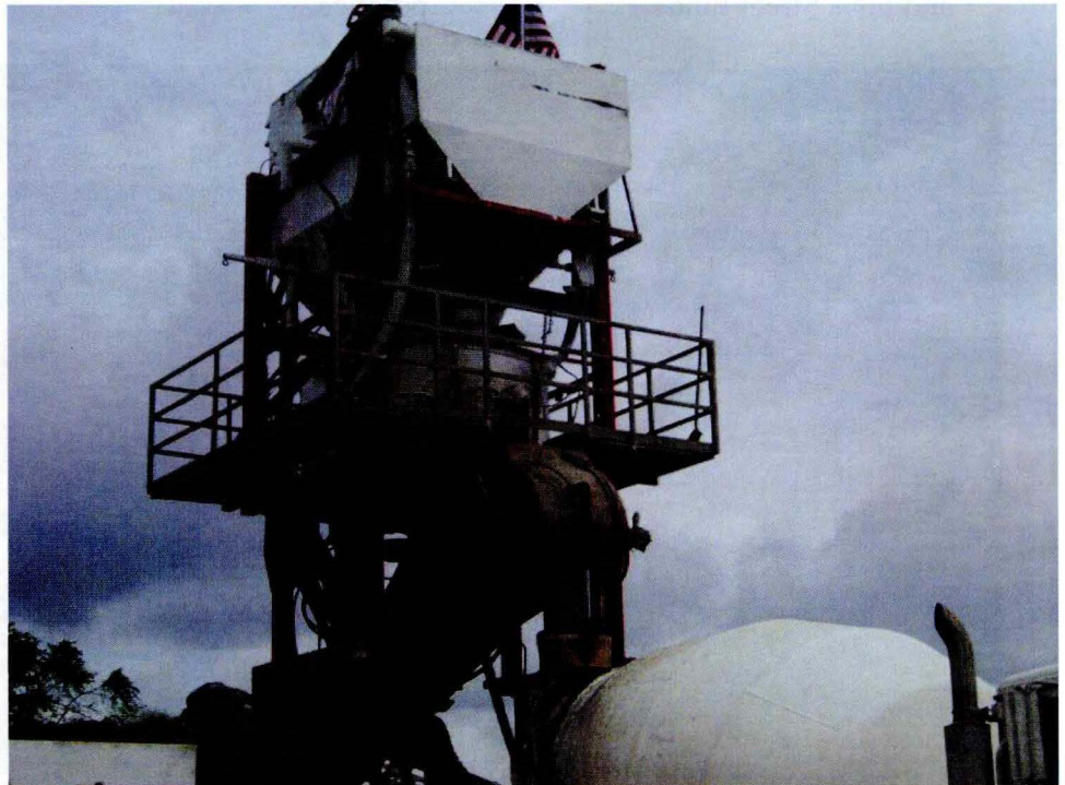
A two stage PCC mixing tower
