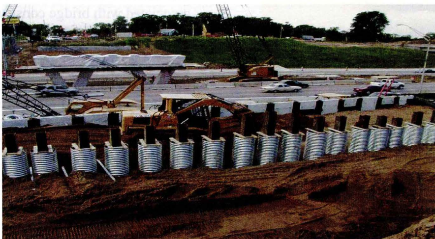
Abutment piles behind a MSE wall for a bridge over I-235 in Des Moines, IA
