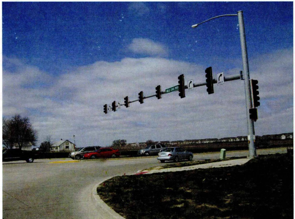
SUDAS specifications are being updated to stay current with new traffic signal technologies and methods used today.
