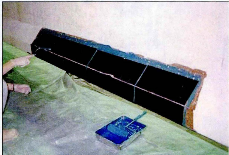
A transverse CFRP jacket being installed on a beam Photo: Iowa State University/InTrans
