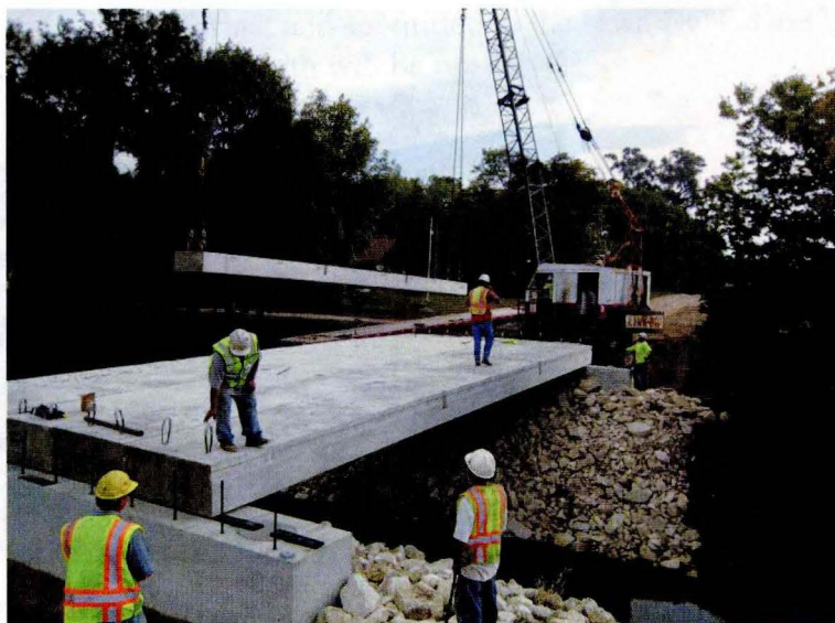
Beam placement during accelerated construction of Buena Vista IBRD bridge Photo: Dr. F. Wayne Klaiber, Iowa State University/CCEE
