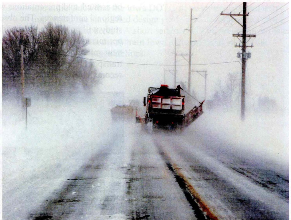
Iowa DOT Maintenance Operations snow removal during a winter storm Photo: Iowa DOT
