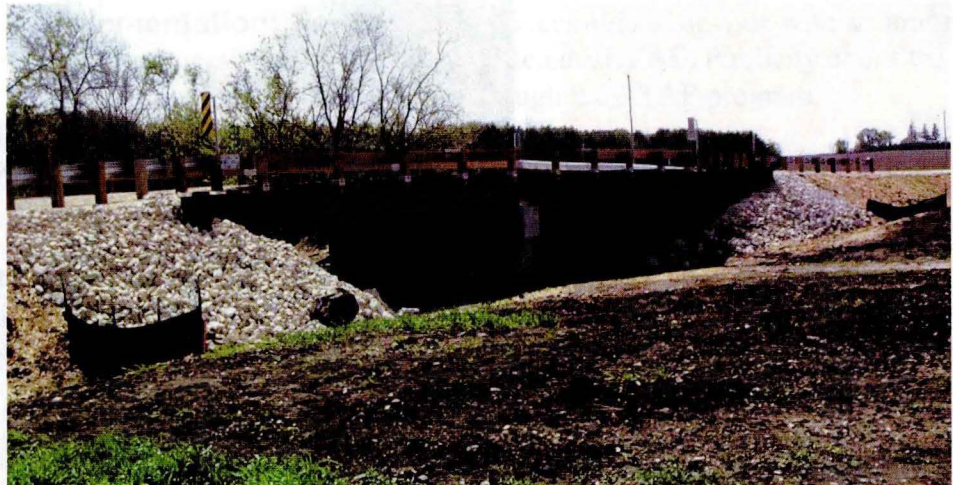
Demonstration timber bridge completed in spring 2009, Delaware County, Iowa, features an innovative deck treatment system
