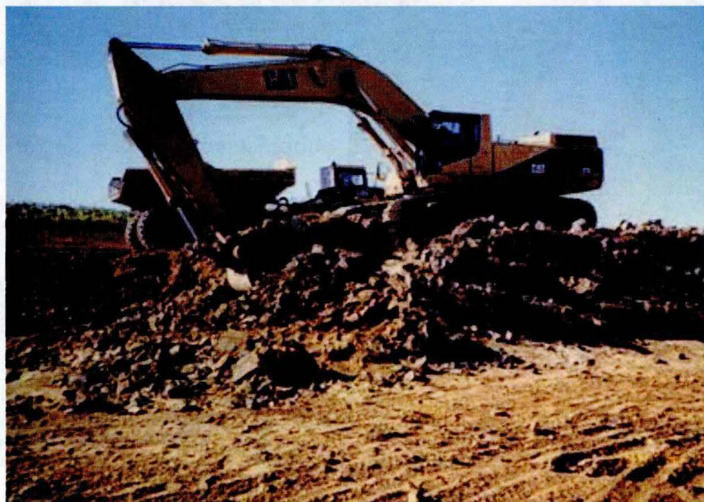
Soil mixing operation through layered soils, Des Moines, Iowa Photo: Vern Schaefer, Iowa State University/CCEE
