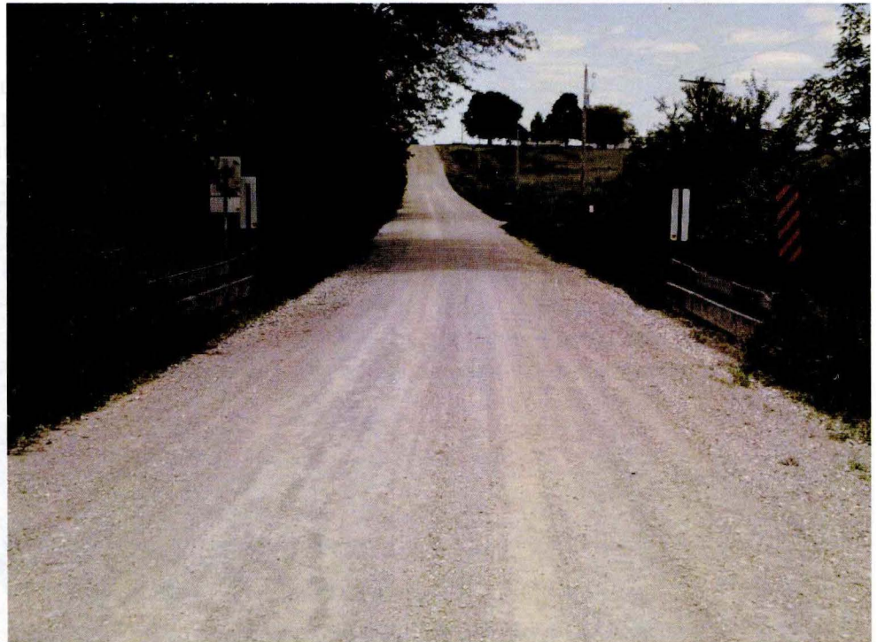
Example of a non-standard timber bridge rail located on a very low-volume road in Central Iowa, June 2009
