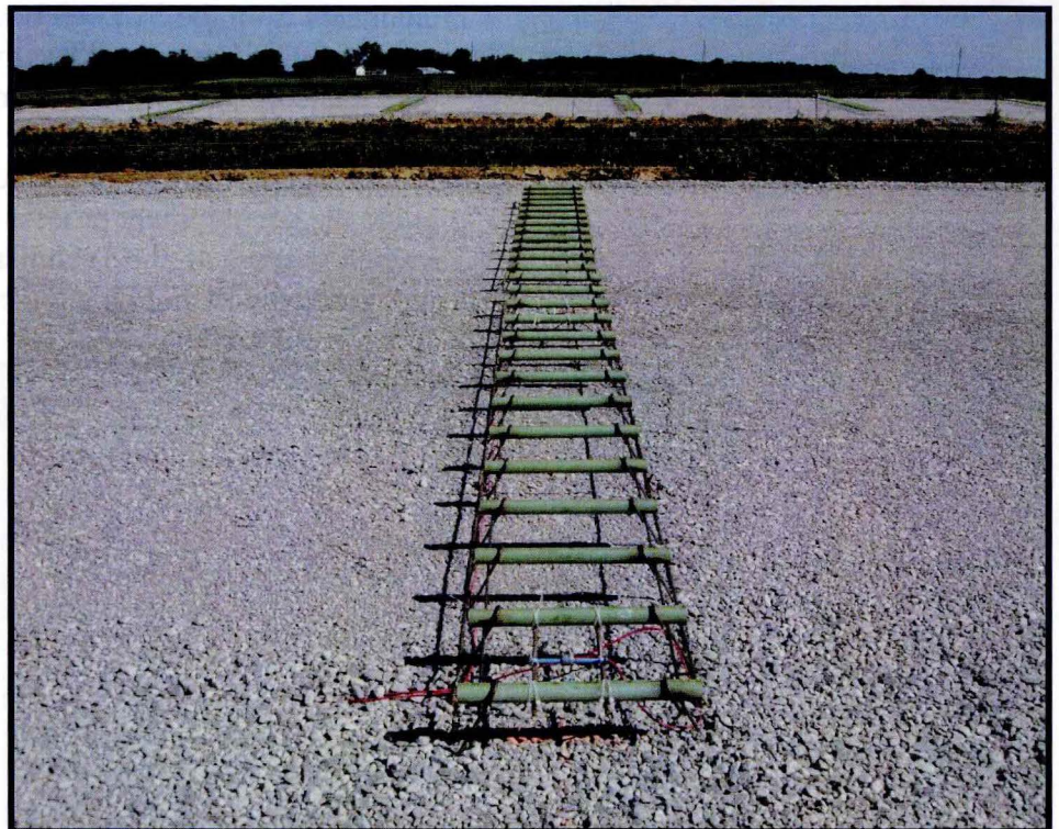
Strain gages installed at joints just before paving monitor stress resulting from concrete shrinkage (US 34 Fairfield bypass)
