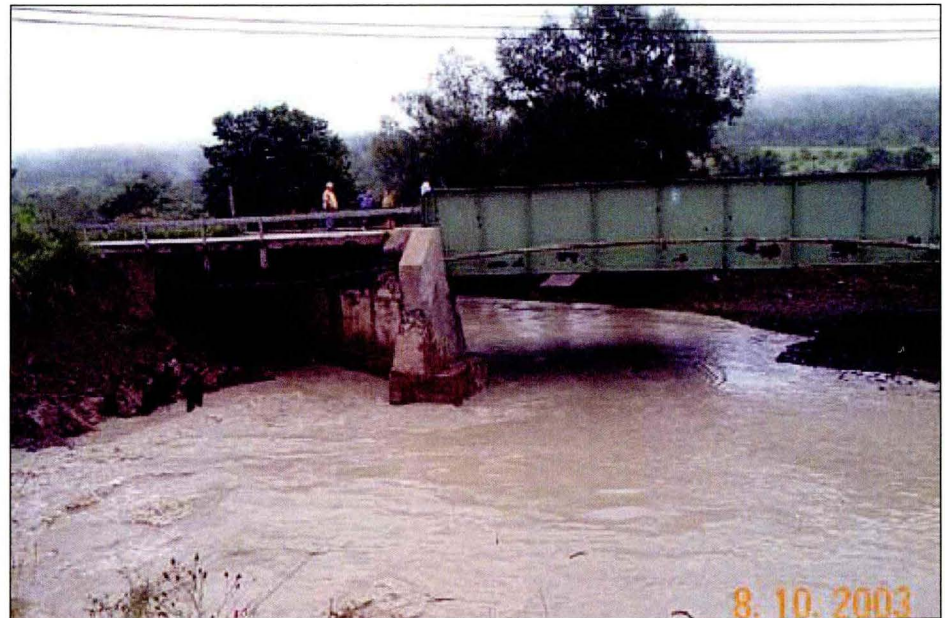
Waterway scour threatens bridge abutment and embankment.
