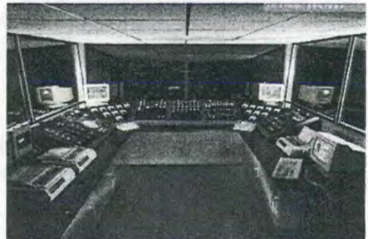
Modern, Computerized Drum-Mix Control
