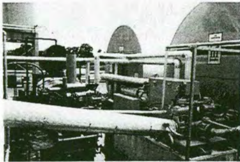
Hot Oil Pipes for Asphalt Tanks
