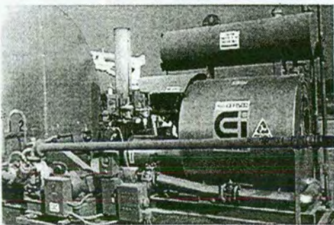
Hot Oil Heater to Heat Asphalt Tanks
