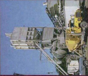
Cement/Fly ash Silos & Weigh Hopper
