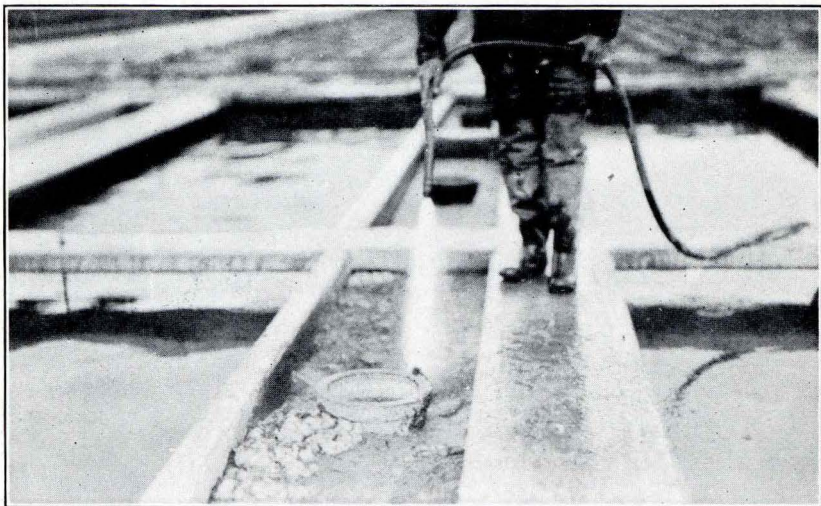
FIG. 5—Hosing the gas-vent chamber of an Imhoff tank to break up the scum layer. This will allow the gas to escape and the solids to settle into the sludge compartments.
