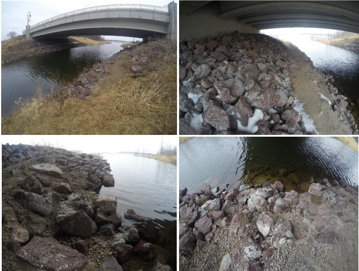
Figure 17. Minnesota Site 2: Partially grouted riprap
