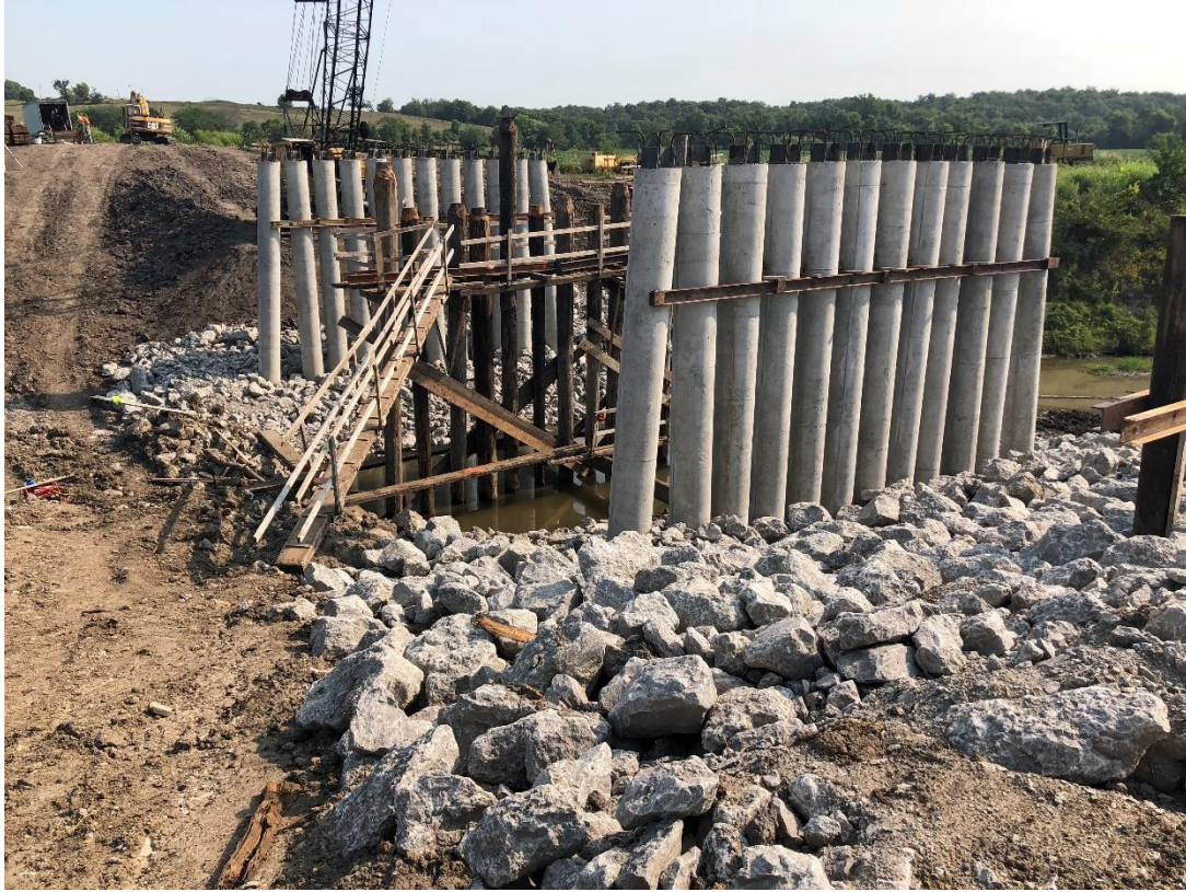
Figure 40. Wayne County pilot installation site
