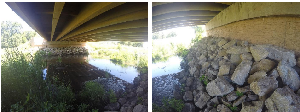
Figure 26. Loose riprap in Buchanan County, Iowa
