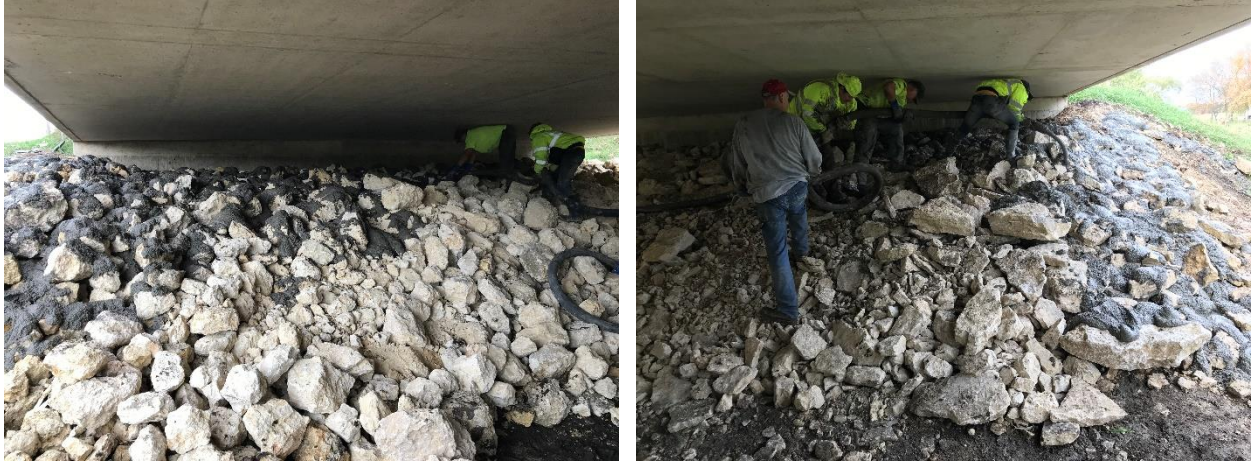
Figure 33. Grouting of Class E revetment (left) and shotrock (right) used for Bridge 1 in Buchanan County
