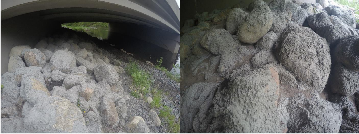
Figure 19. Minnesota Site 4: Partially grouted riprap—splash of grout
