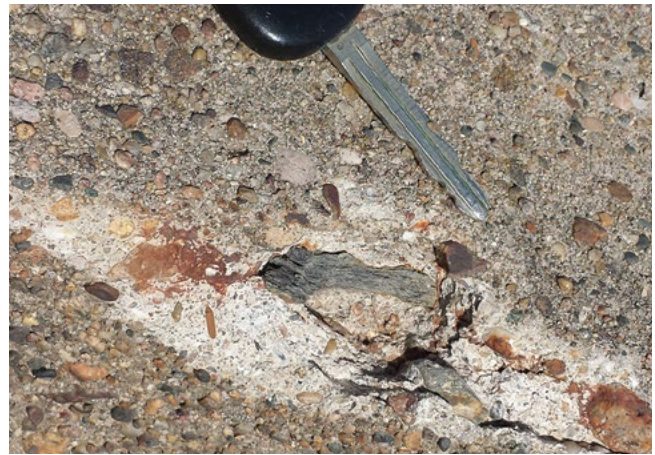
Figure 4-14. Popout at the concrete surface
